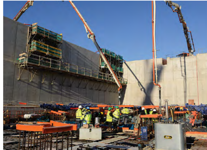
Pouring the first plot of the upper basemat of the Tokamak complex (December 2013)
