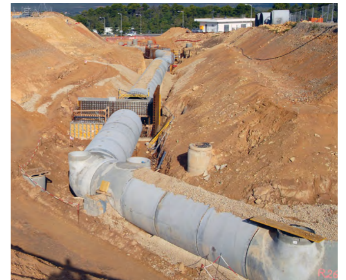
Precipitation drainage system
