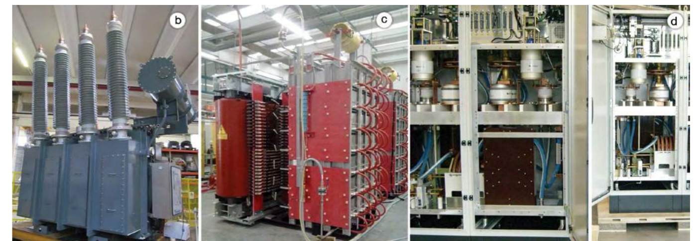
a. The ISEPS power supplies are hosted on a 12 x 10 m insulated platform. They are fed and insulated at -100kV from ground via an insulating transformer (22kV/6.6kV, 5MVA) located outdoors, (Image courtesy of OCEM).
