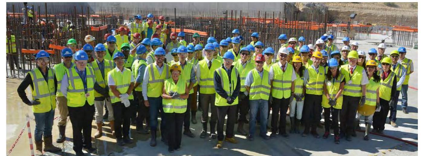
Hundreds of workers have been involved in the construction of the B2 Slab.
