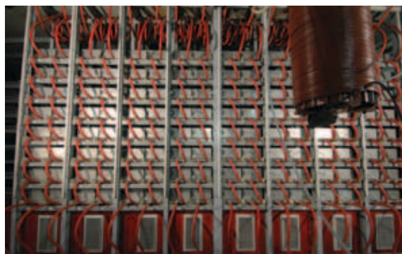
The main High Voltage power supply for the 2MW European gyrotron for ITER installed at the European Electron Cyclotron Test Facility at CRPP (Lausanne, Switzerland), and successfully tested at full power on dummy load in 2009. (Image courtesy of OCEM)
