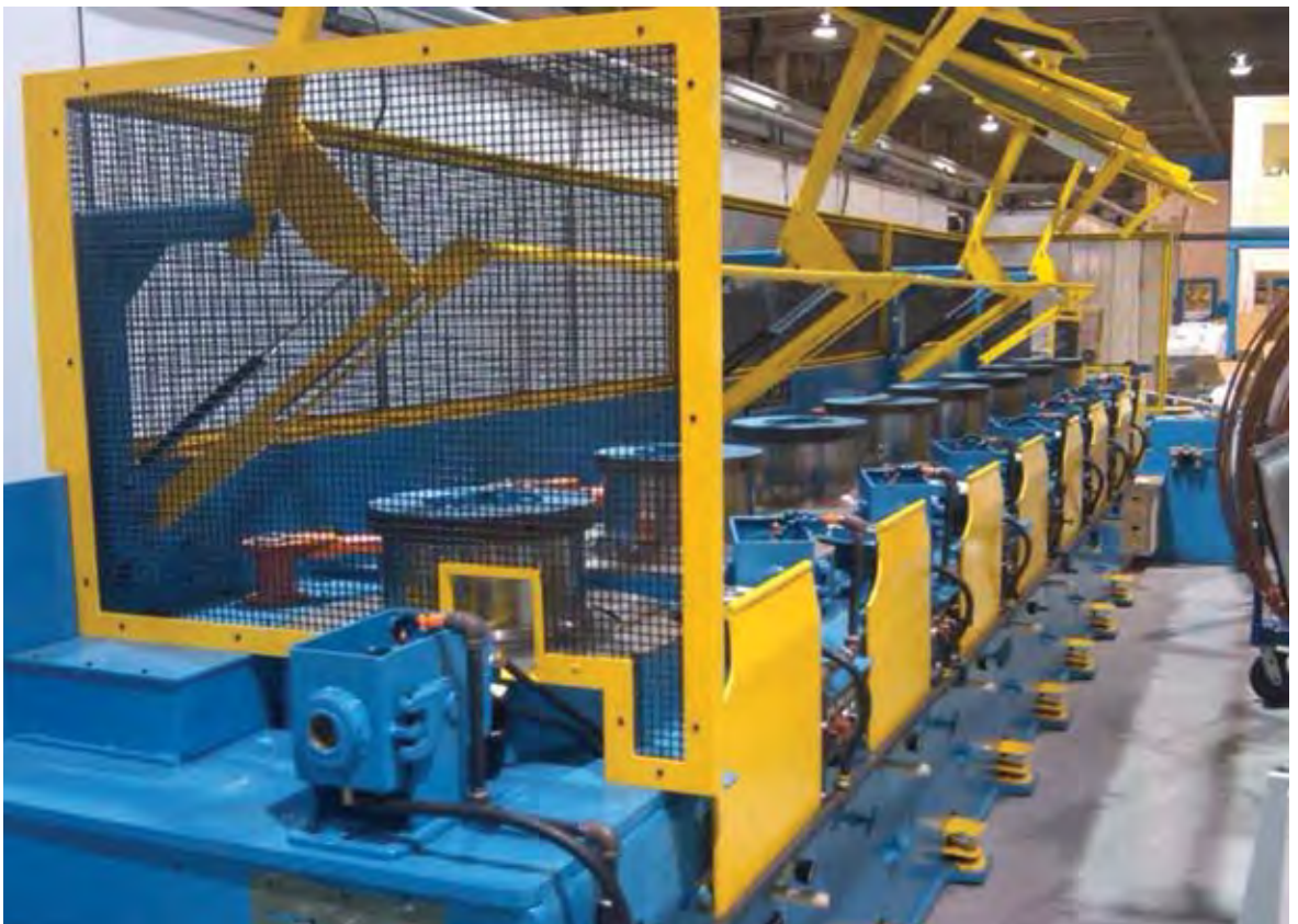
Fig. 7: Manufacturing facility for Nb 3 Sn strand drawing (courtesy of OST)
