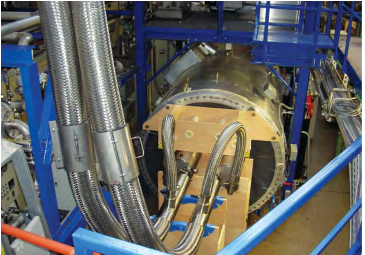
Fig. 13: View of TIMO-2 Facility at KIT being upgraded to provide 4.35 K supercritical He for testing the ITER Torus Cryopumps (courtesy of KIT)
