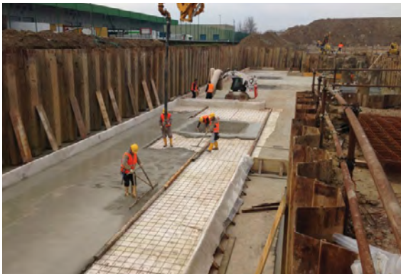
Water basins for the cooling plant at the PRIMA site
