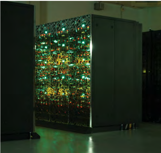
The supercomputer Helios in operation: Helios dissipates nearly 3MW when working at full power.
