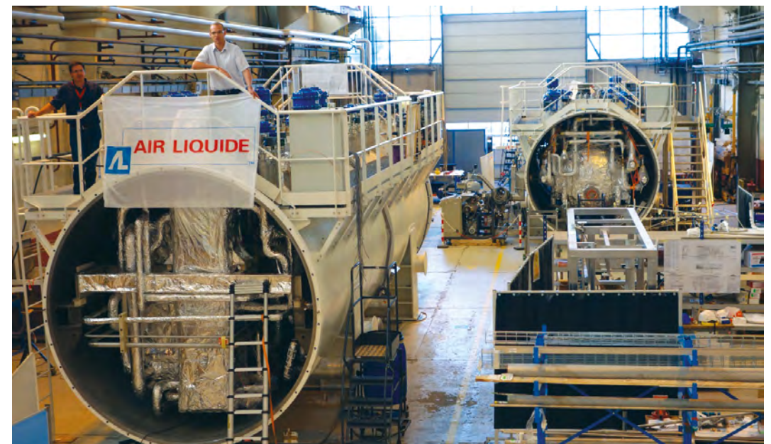
Refrigeration cold boxes (cold end) with insulated cold components
