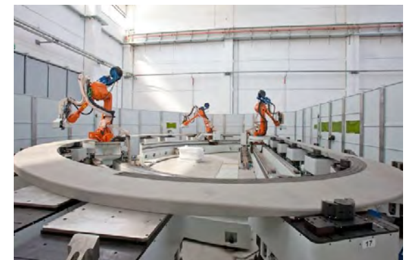
The laser welding machine in operation during welding of cover plates on a side DP in ASG, La Spezia (Courtesy of CON)
