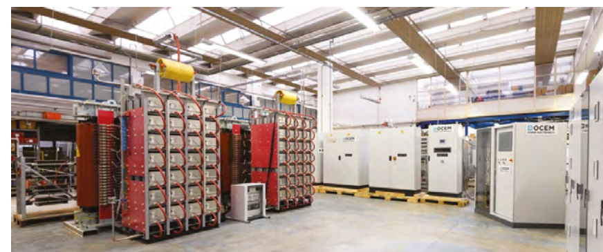
Layout configuration for the full Factory Acceptance Testing of ISEPS of SPIDER at OCEM Energy Technology premises Padova site (Consorzio RFX premises)
