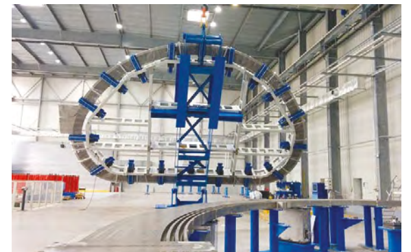
In the background a radial plate is being flipped at SIMIC. In the foreground a pre-machined side radial plate waiting to be transferred to the portal machine for the final machining (courtesy of CSC).
