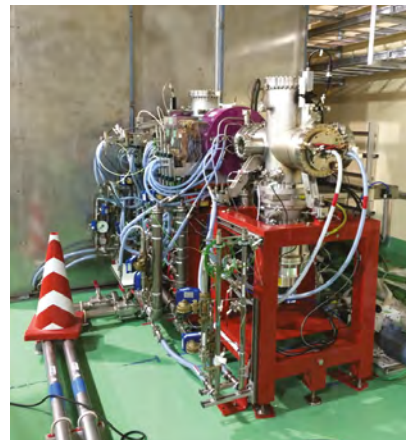
The injector of the LIPAc accelerator installed in Rokkasho
