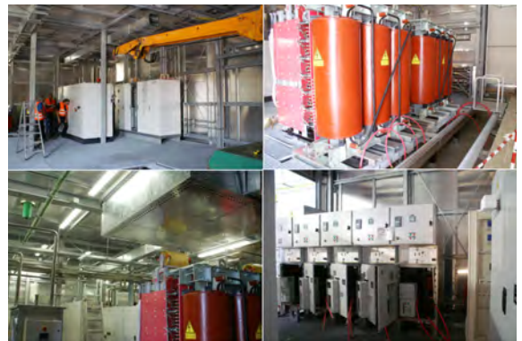
The ISEPS installation at the NBTF site in Padua, Italy
