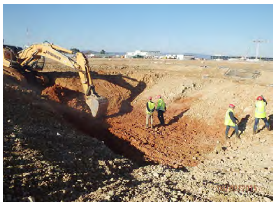
The Transformers' area in March 2015
