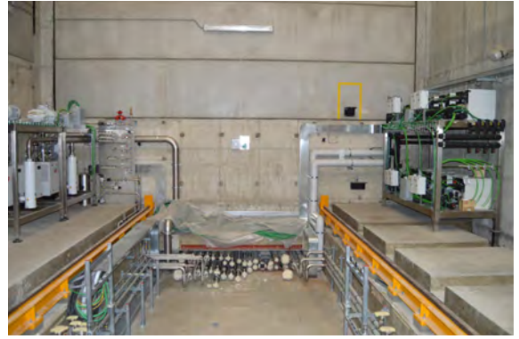
General overview of on-going installation of the vacuum system inside the SPIDER bio-shielding
