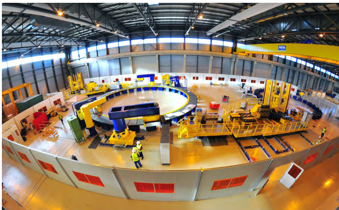
PF 2-5 Winding Machine installation in the PF Building at the Cadarache site
