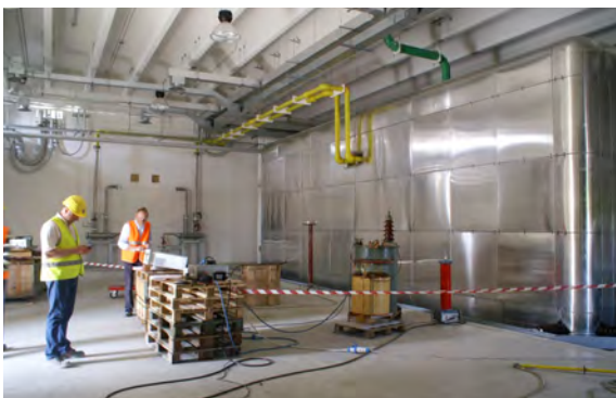
The SPIDER High Voltage Deck during tests
