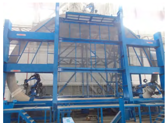
The three big sectors of the Radial Plate are being welded in the welding frame at the SIMIC site (Courtesy of SIMIC)
