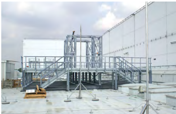
Installation of the cooling towers on top of the roof of Building 2 at the NBTF
