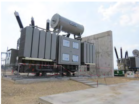
The installed transformers in August 2015
