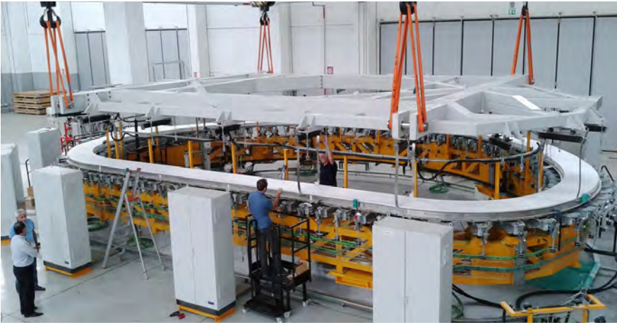
Assembly of a series DP on the VPI mould, ready to be impregnated in ASG, La Spezia (Courtesy of ASG)
