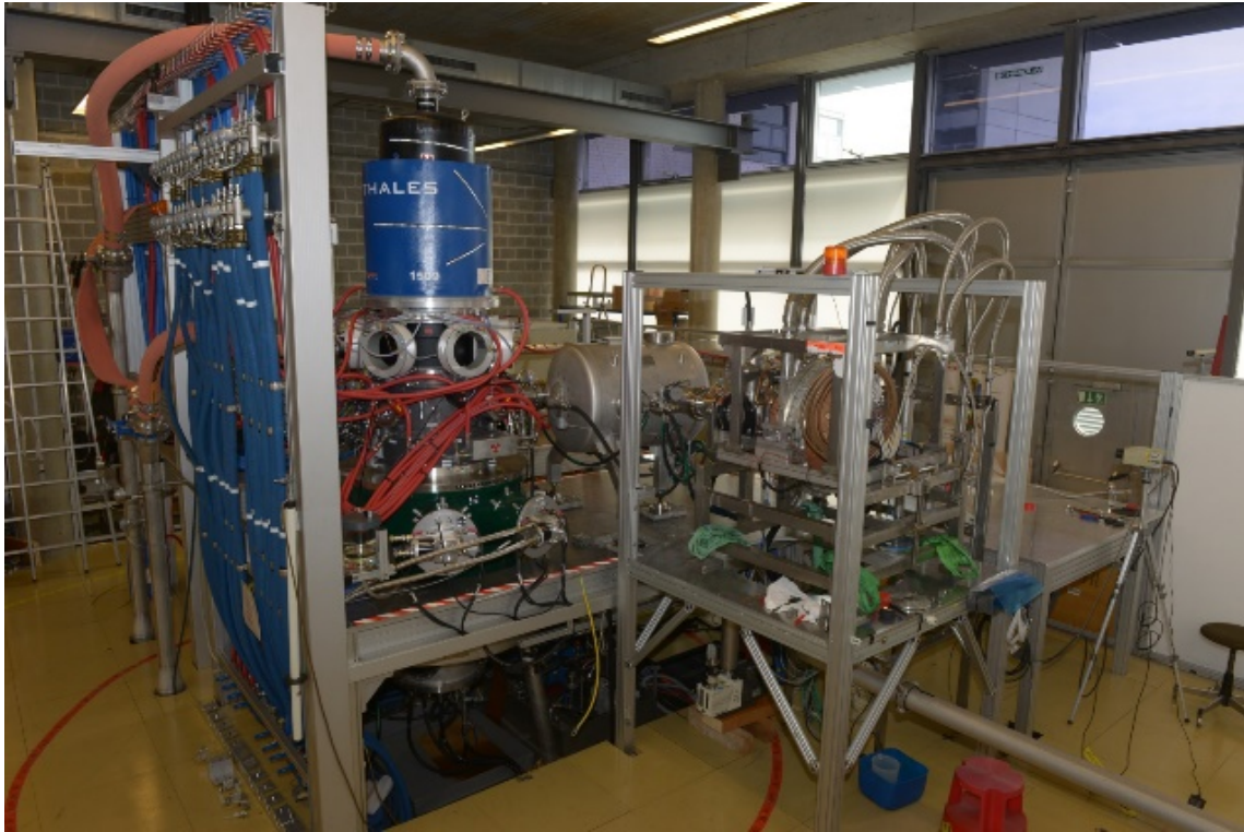
Figure 14: The prototype 1MW European gyrotron installed undergonig test in the new "Falcon" facility at the Swiss Plasma Center in Switzerland
