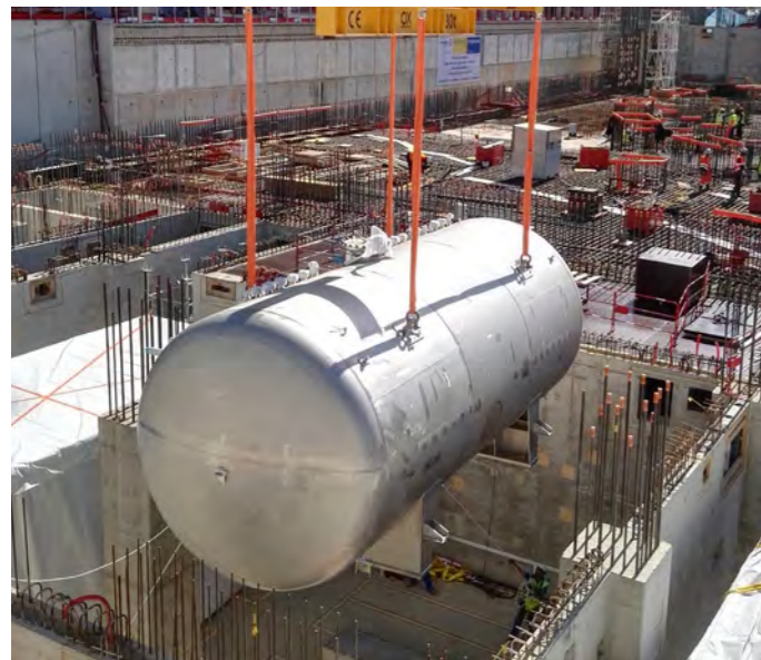
Transferring one of the bigger water detritiation tanks weighing approximately 20 tonnes in ITER's Tritium building
