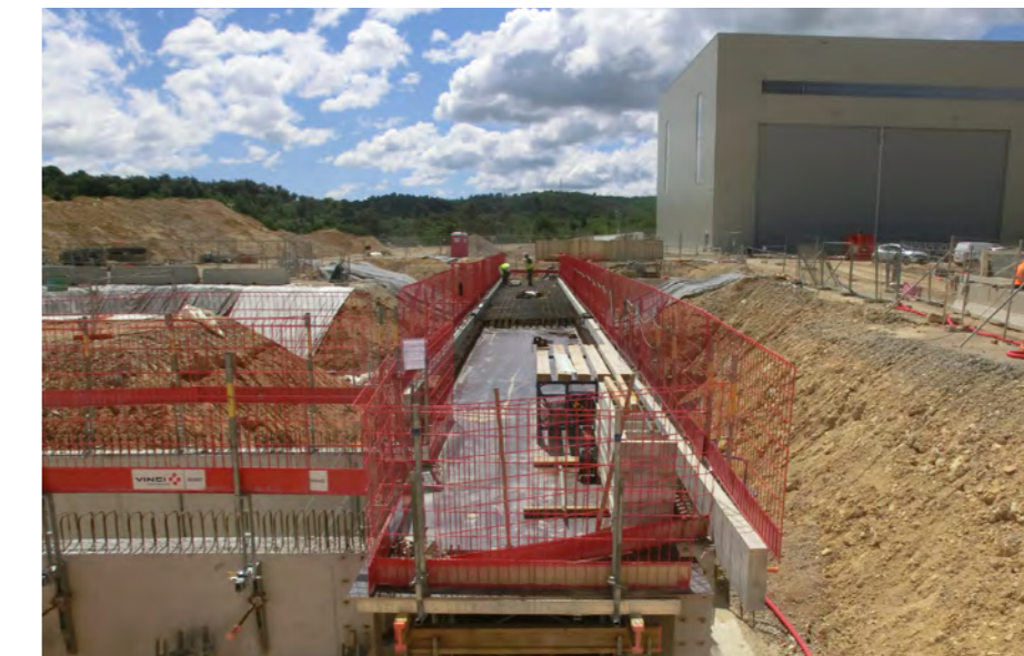
The ITER site galleries under construction that will enable the connection of necessary services between buildings, June 2016 © F4E
