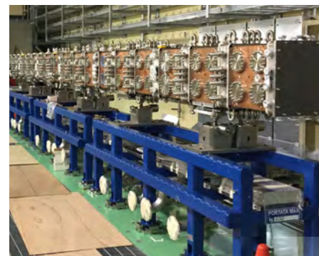
Installing the Radio Frequency Quadrupole and Injector already in position in Rokkasho, IFMIF/EVEDA, Rokkasho, Japan.
