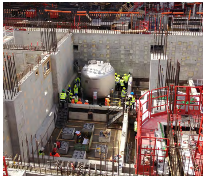
Installing one of the smaller water detritiation tanks weighing approximately 5 tonnes in ITER's Tritium building
