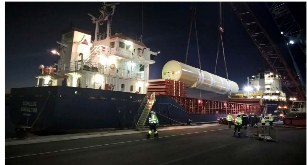
Unloading the second quench tank at Fos-sur-Mer, the port of Marseille, November 2016
