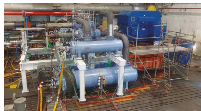
Nitrogen compressor of the ITER LN2 plant successfully tested at Atlas Copco
