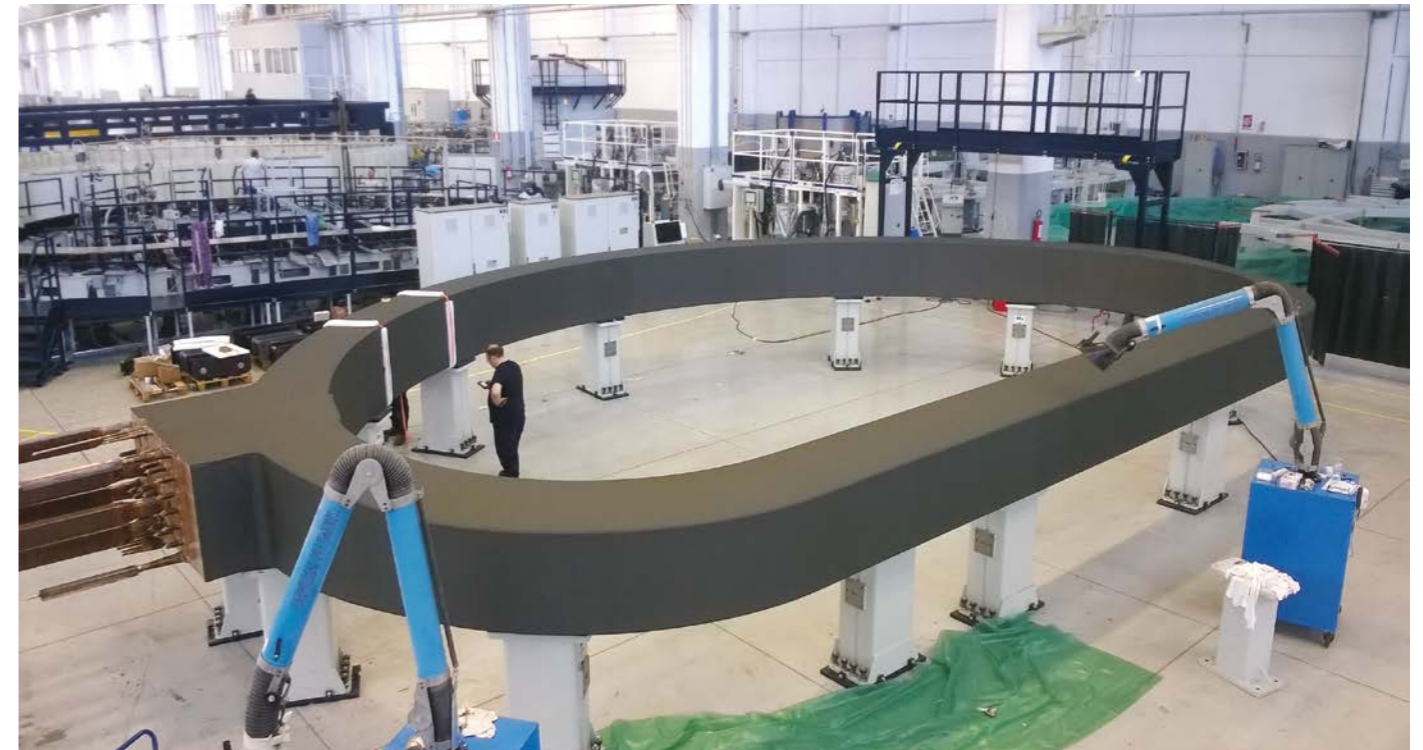
Applying special conductive paint to the surface of the winding pack, ASG Facility, La Spezia, Italy
