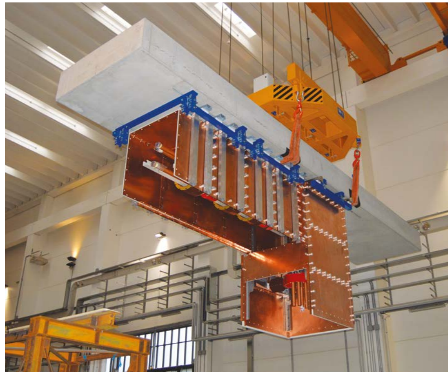
Part of the 35 metre long transmission line which is connected to the SPIDER vessel
