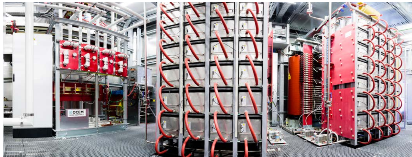
The Ion Source and Extraction Power Supply (ISEPS) for the SPIDER test bed (photos courtesy of OCEM ET)
