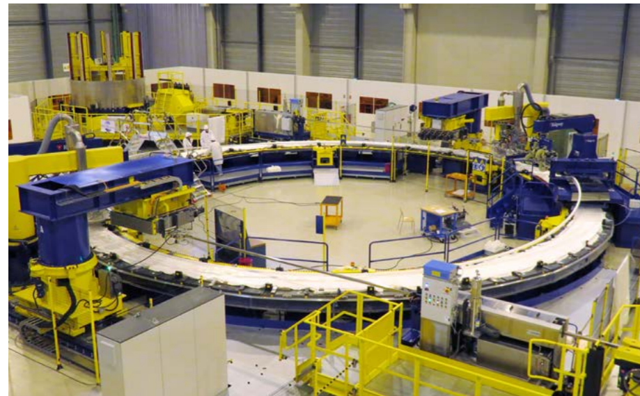
The first complete layer using a dummy conductor reflecting the dimensions of ITER's fifth Poloidal Field coil, Cadarache, November 2016
