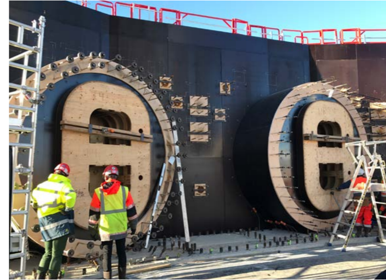
The entry points of the ITER Neutral Beam Injectors at the second floor of the Bioshield, Tokamak Complex, December 2016, © Engage
