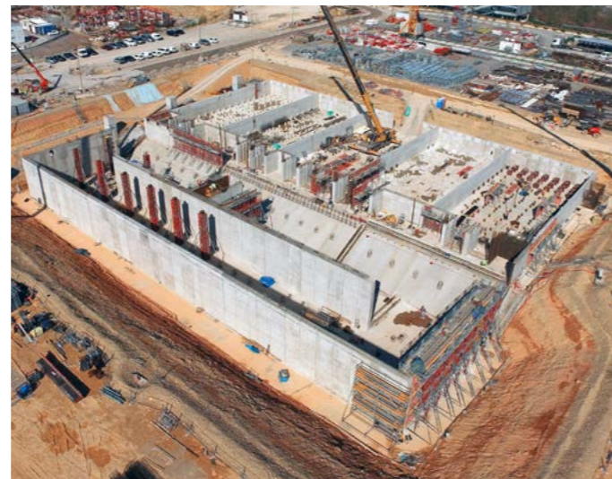
Civil engineering works progressing at the water basin and cooling water stations of the ITER device, April 2017, © E. Riche/ITER Organization
