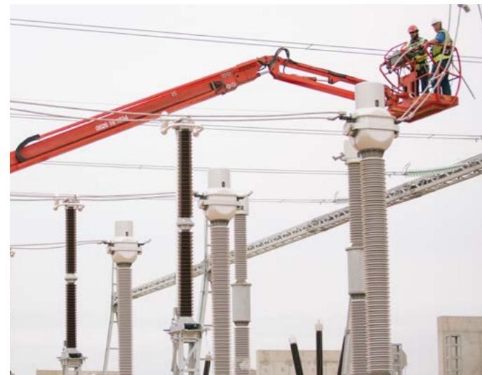
Technical teams checking the cabling where the ITER substation will be connected to France's grid to receive 400 kV, November 2016, © LNM
