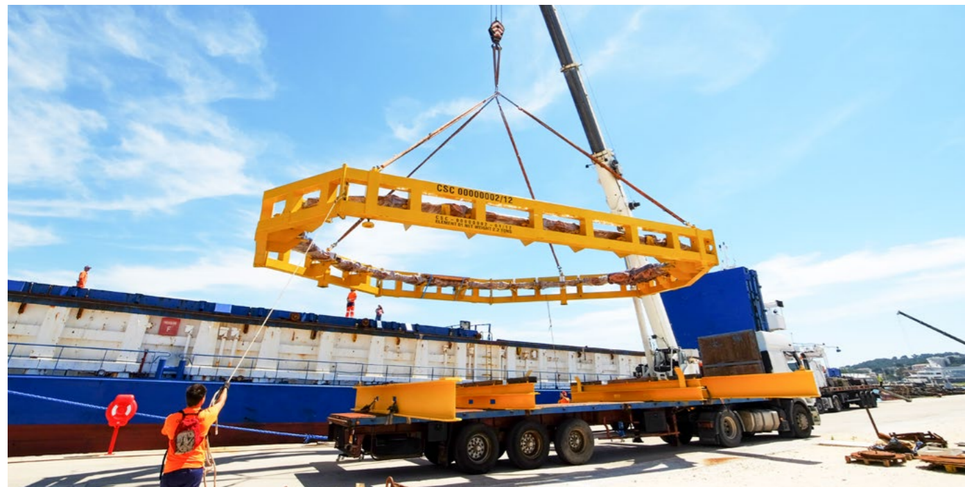
Loading Europe's last radial plate manufactured by CNIMTED on behalf of F4E
