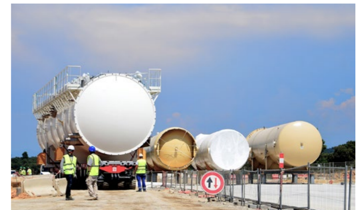
(L-R) Helium Plant Cold box stationed next to the gaseous helium (GHe) tanks and the liquid nitrogen (LN2) tank on-site, Cadarache, June 2017 © ITER IO
