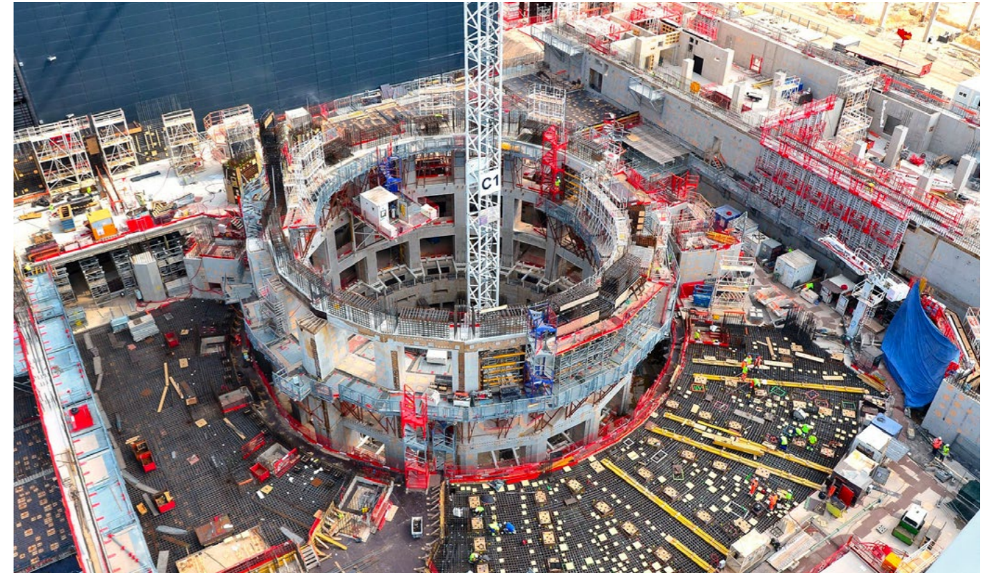
Civil engineering works progressing at the bioshield, ITER site, June 2017 © ITER IO
