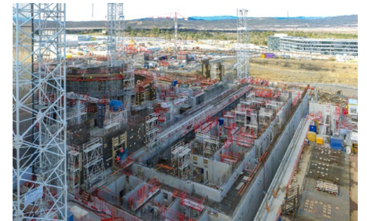
The progress of the slab and walls of the ITER Tritium building, April 2017 © LNM
