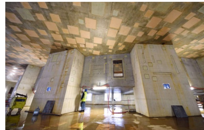
The embedded plates can be viewed on the level above © ITER IO
