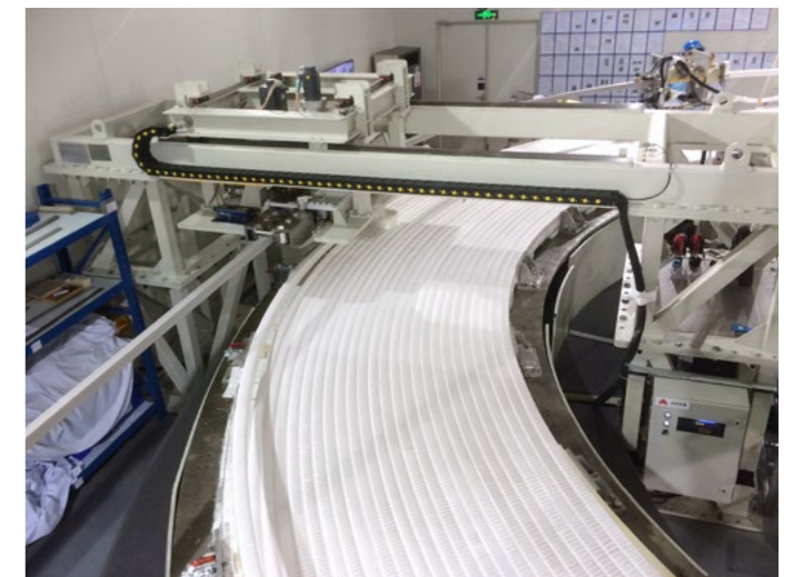
The Winding of the first Double Pancake of Poloidal Field coil 6 has been completed, ASIPP, China
