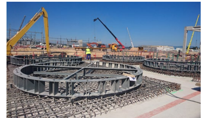
The embedded anchors indicate the exact positions where the tanks need to be installed on-site, Cadarache, June 2017 © Engage
