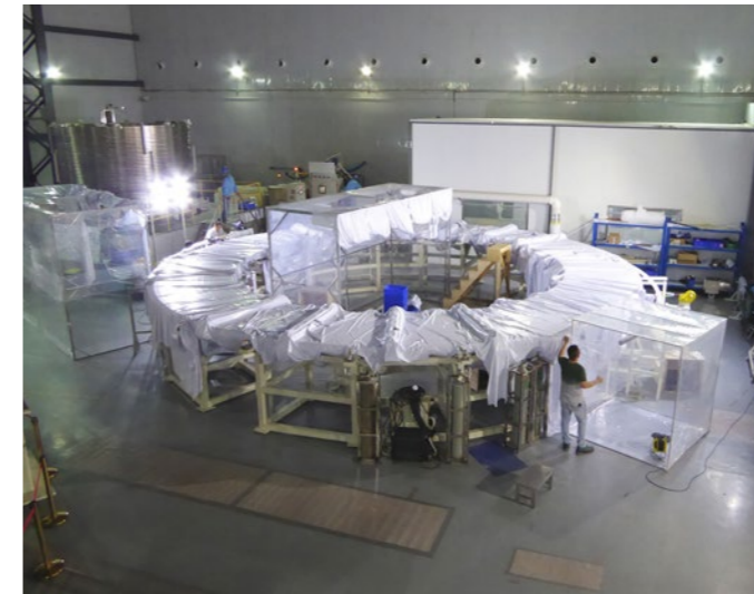
Working on the terminations of one Double Pancake of Poloidal Field coil 6, ASIPP, China
