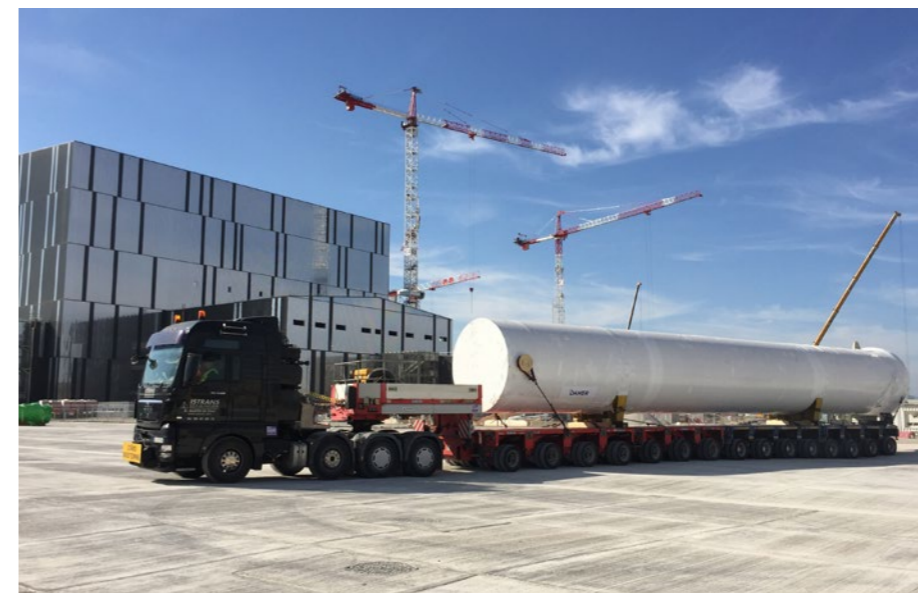
The GN2 buffer tank, part of ITER's Cryogenic system, has been delivered on-site, Cadarache, October 2017
