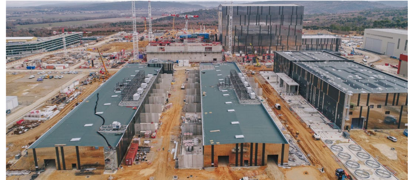
(L-R) Aerial view of the two ITER Magnet Power Conversion Buildings and the ITER Cryoplat, December 2017 © SNC Engage
