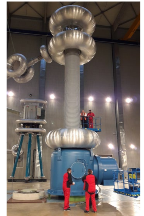
The installation of the High Voltage Deck inside the MITICA High Voltage hall, October 2017. © Consorzio RFX
