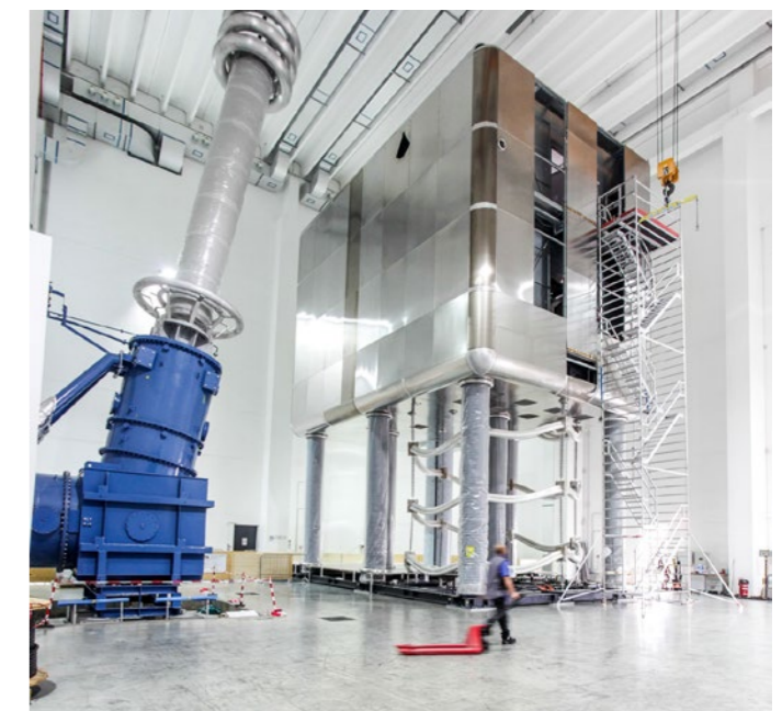
The installation of the High Voltage Deck inside the MITICA High Voltage hall, October 2017. © Consorzio RFX
