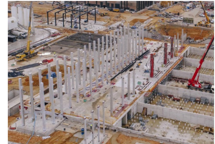
Starting to plan the installation of equipment at the ITER Cold Basin and Cooling Towers facility, December © SNC Engage
