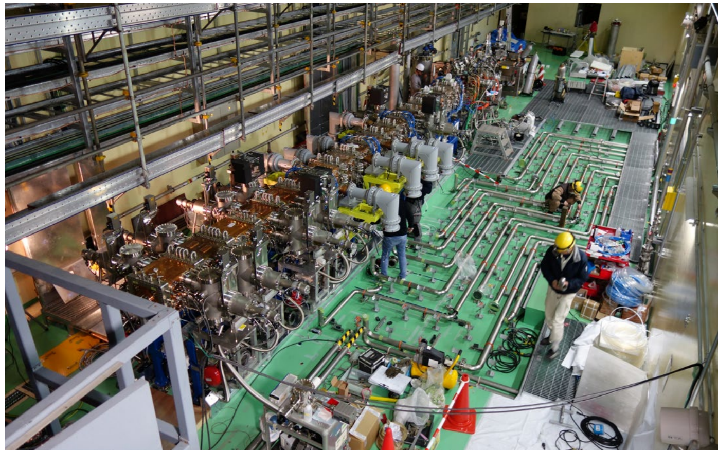
Top view into the LIPac accelerator vault during the installation of the cooling loops for the "Radiofrequency Quadrupole", Rokkasho, Japan
