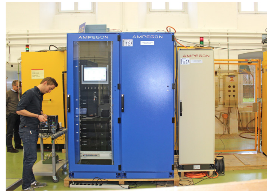
F4E and Ampegon checking the equipment during testing © F4E
