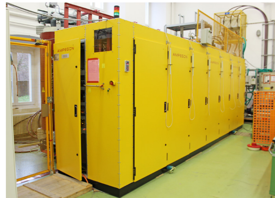
High voltage power supply unit financed by F4E and manufactured by Ampegon © F4E
