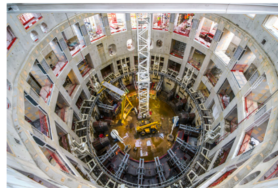
View of the ITER Bioshield lid, positioned 30 m high, ITER construction site, Cadarache, March 2018 © ITER IO
