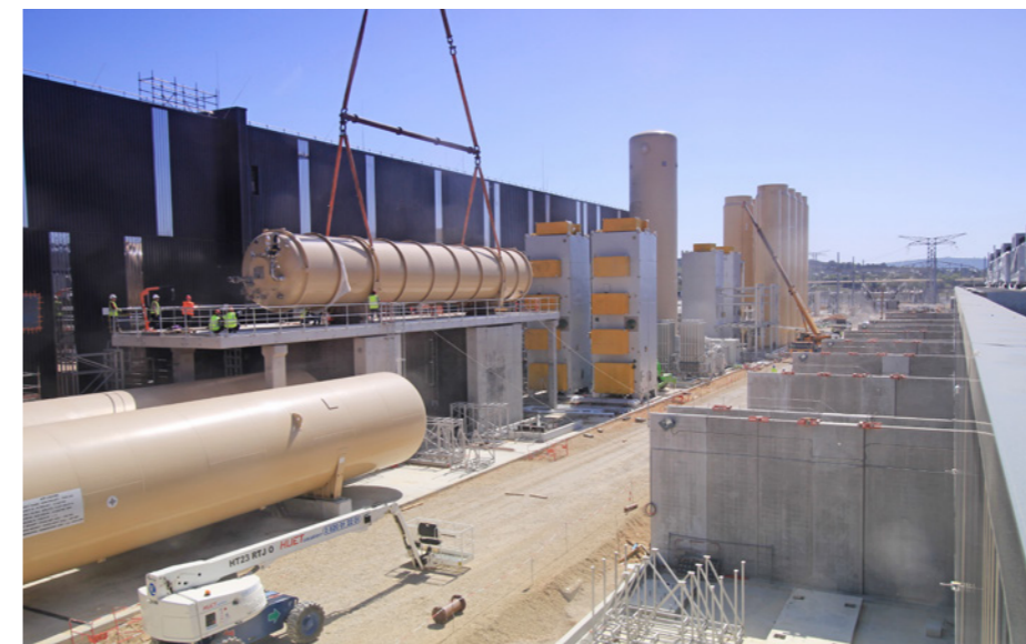
More components produced by Europe have been installed on-site: the two quench tanks on the ground, the LHe tank on the level above, and the cold boxes. At the far end the remaining cryogenic tanks.
