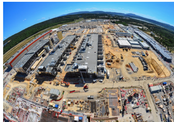
(L-R) Poloidal Field coils facility, ITER Cryoplant, Magnets Power Conversion buildings, galleries civil engineering works on-going, ITER construction site, July 2018 © ITER IO
