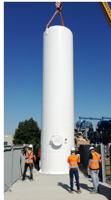
Installation of the Gas Helium tank at ITER Neutral Beam Test Facility, MITICA, Padua, Italy
