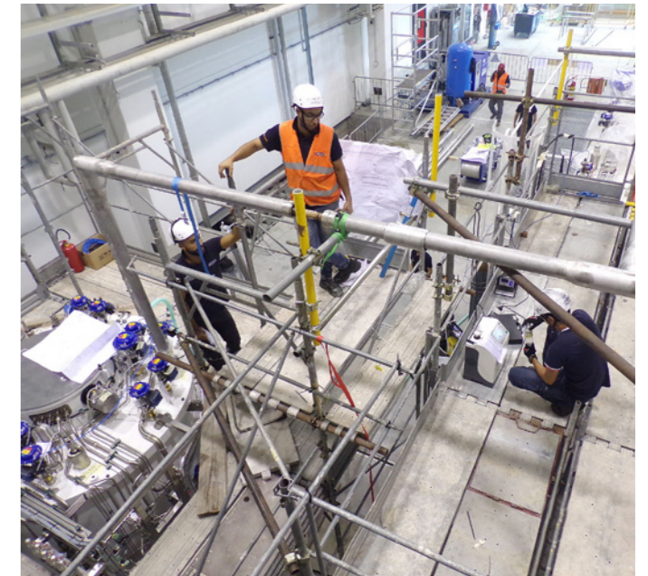
Connecting the main cold box, on the left, with the auxiliary cold box, on the far right, with the help of cryolines, ITER Neutral Beam Test Facility, MITICA, Padua, Italy
