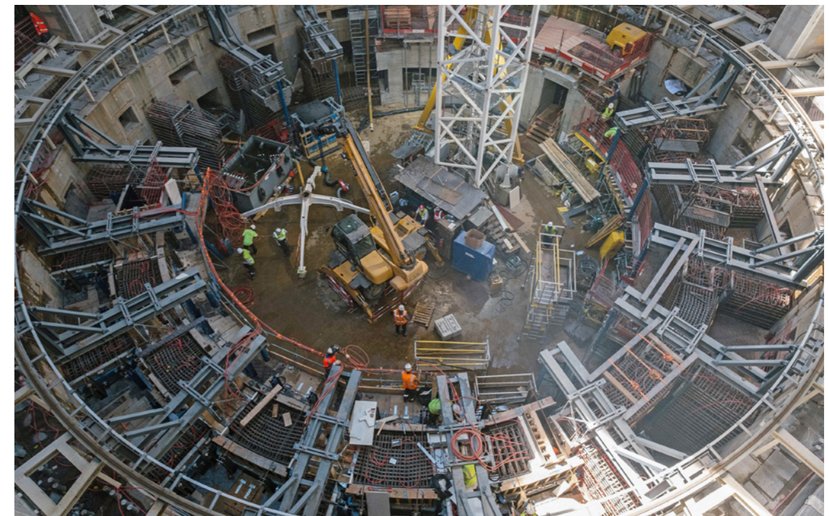
Building the crown that will support the ITER machine, Tokamak building, ITER construction site, Cadarache, June 2018
