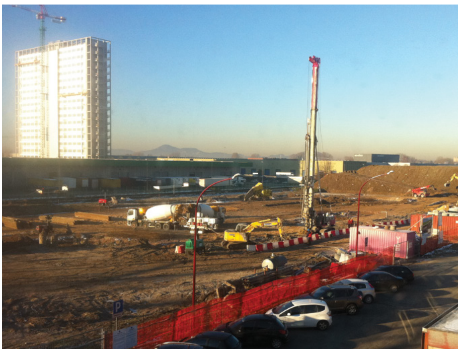
Progress on the NBTF site: The construction of buildings is moving ahead
