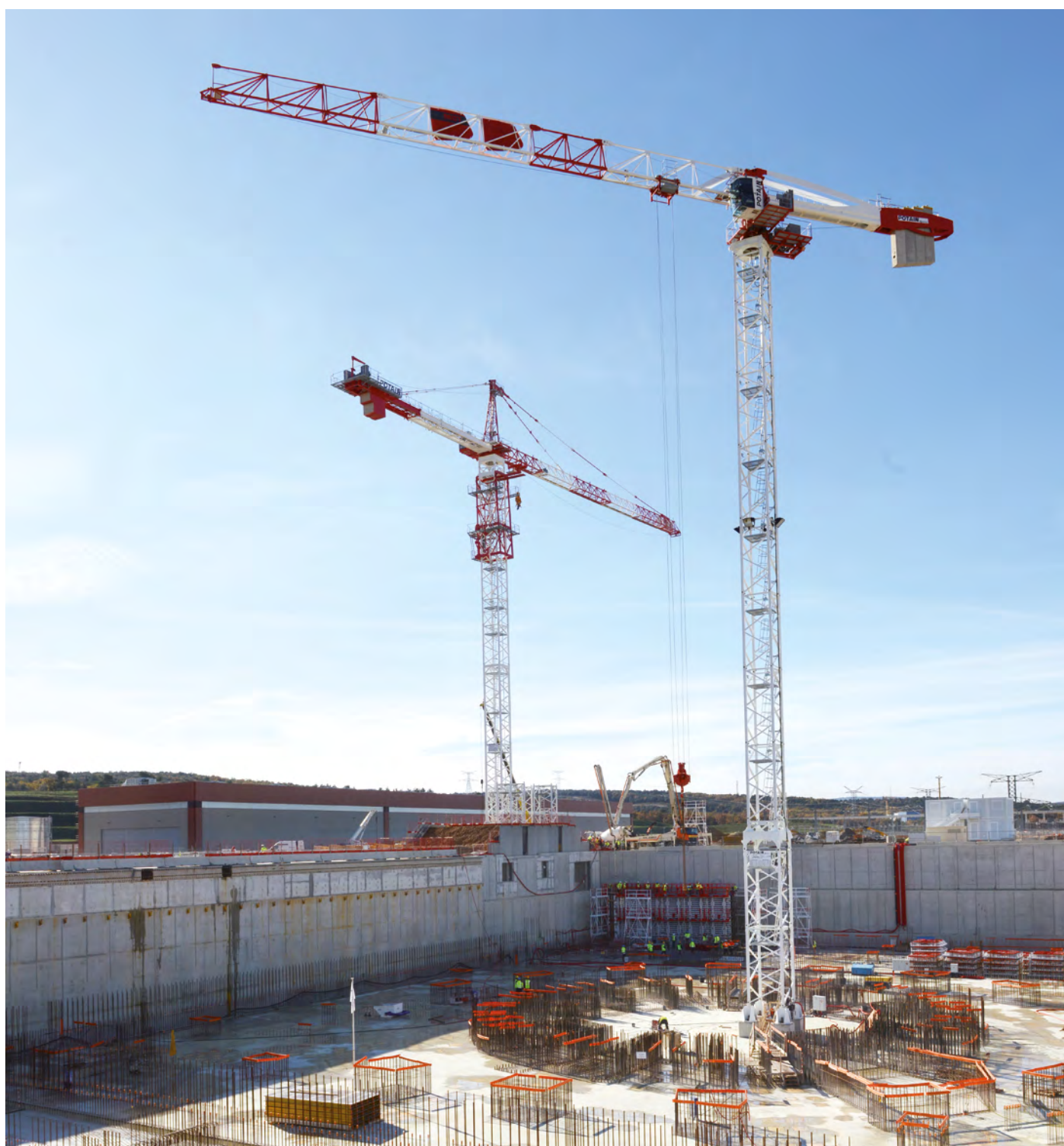
Tokamak complex – The cranes are erected and the concrete is being poured for the First Wall – November 2014
