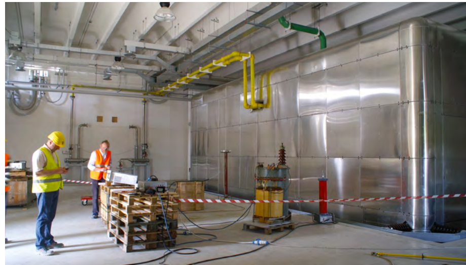
During the acceptance tests of the SPIDER High-Voltage Deck (HVD) at the Neutral Beam Test Facility (NBTF) at the Consorzio RFX site in Padua, Italy.
