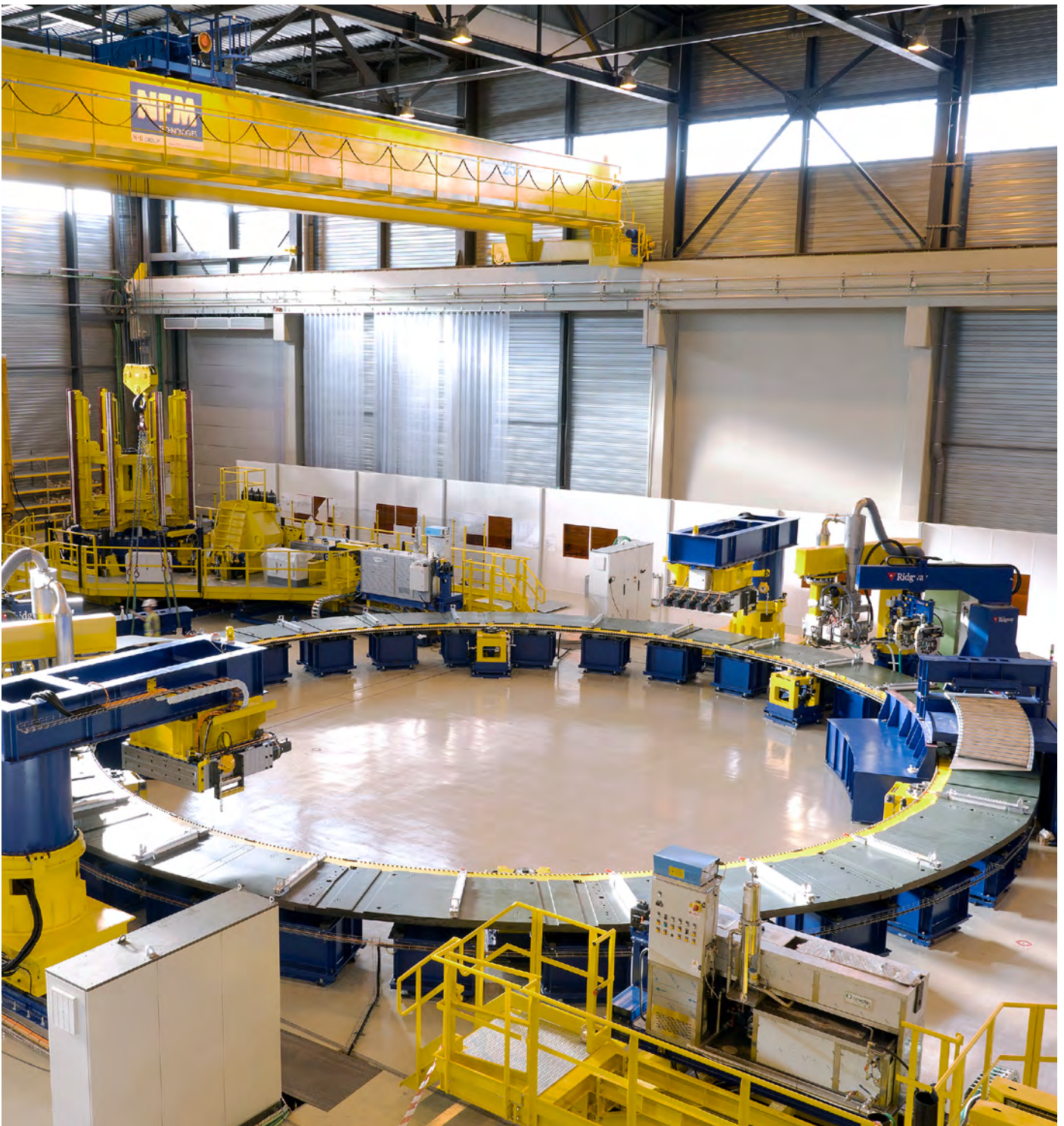
Setting up the conductor winding tooling station, ITER PF Coils facility, Cadarache.
