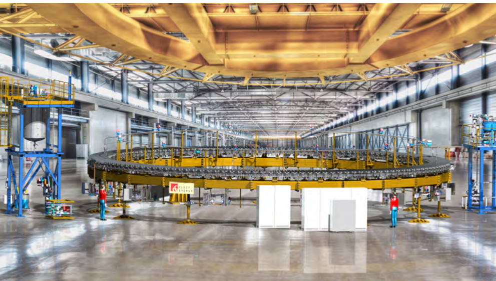
3D image of PF coils tooling station, Elytt Energy / Christian Lünig/ VG Bild und Kunst ©
