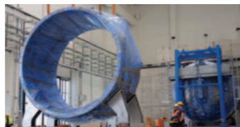
Installation of SPIDER Vacuum Vessel.
