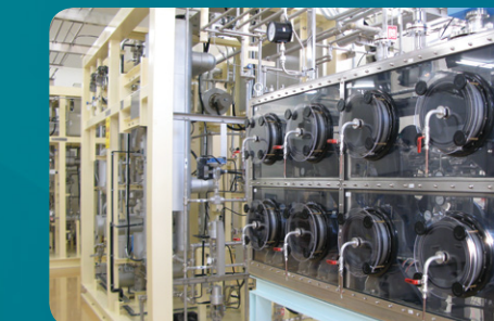
Tritium handling equipment
