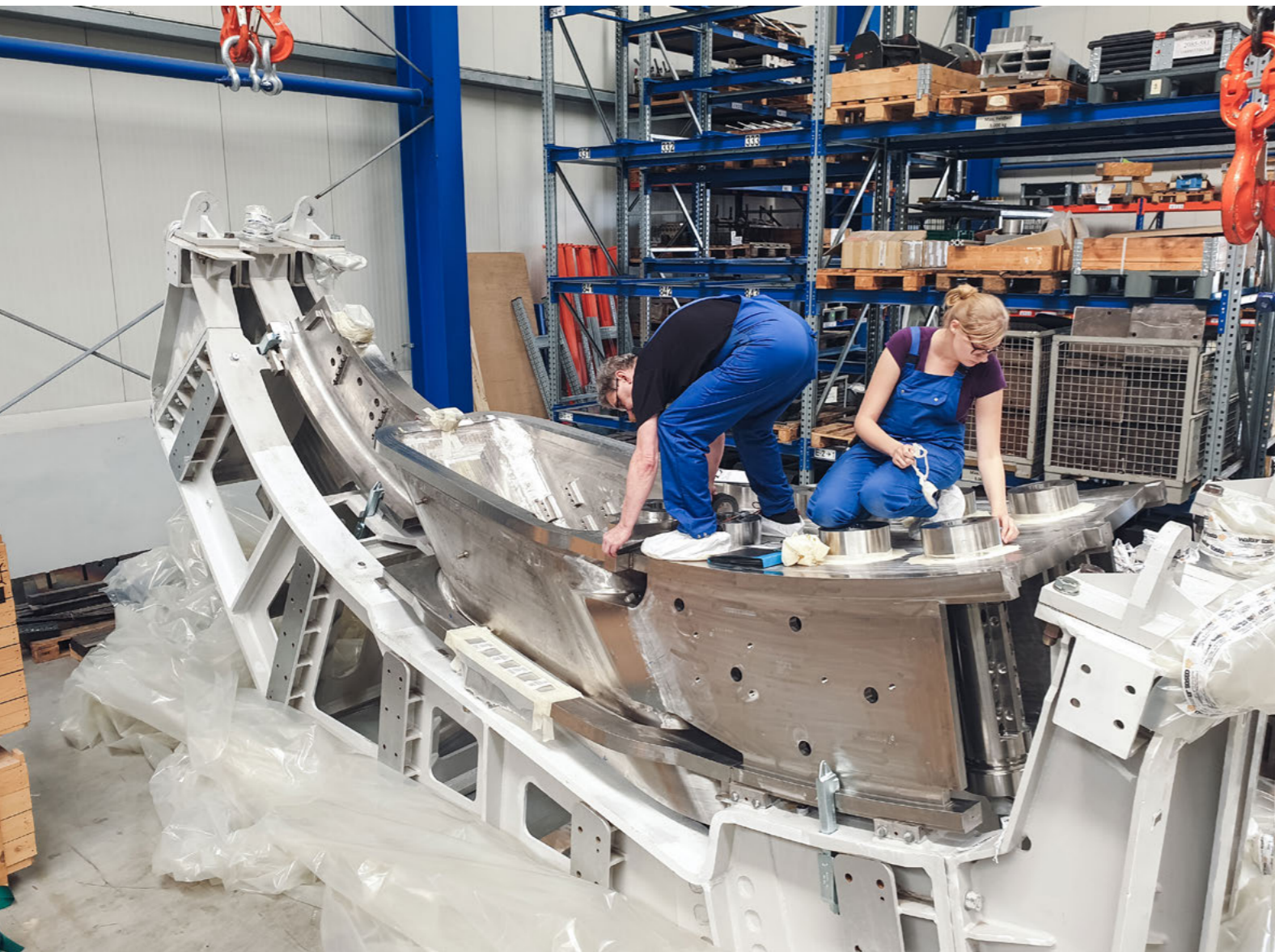
Before welding: Inspection at ProBeam of the last sector 5 assembly with a central port arriving from Walter Tosto.
