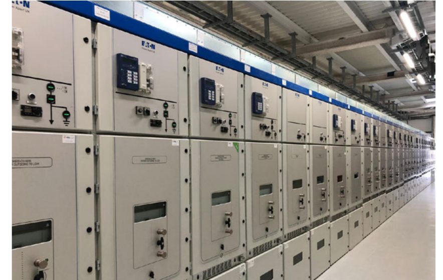
View of the equipment installed in the Power Supplies building. The works have been financed by F4E and carried out by Ferrovial, ITER construction site, Cadarache, France, October 2019 © F4E
