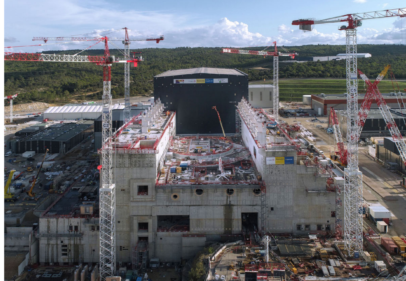
ITER Tokamak Complex during final pouring of concrete, Cadarache, France, November 2019 © ITER Organization/EJF Riche
