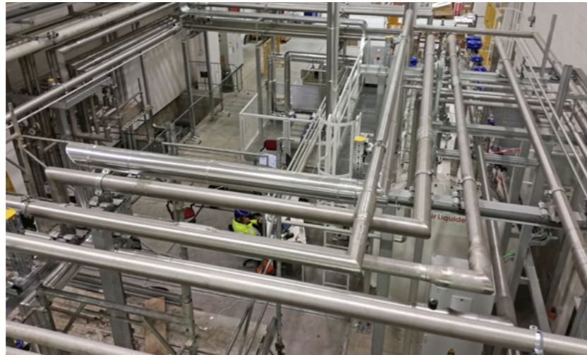
Cryolines connecting the main cold box with the auxiliary cold box, ITER Neutral Beam Test Facility, MITICA, Padua, Italy
