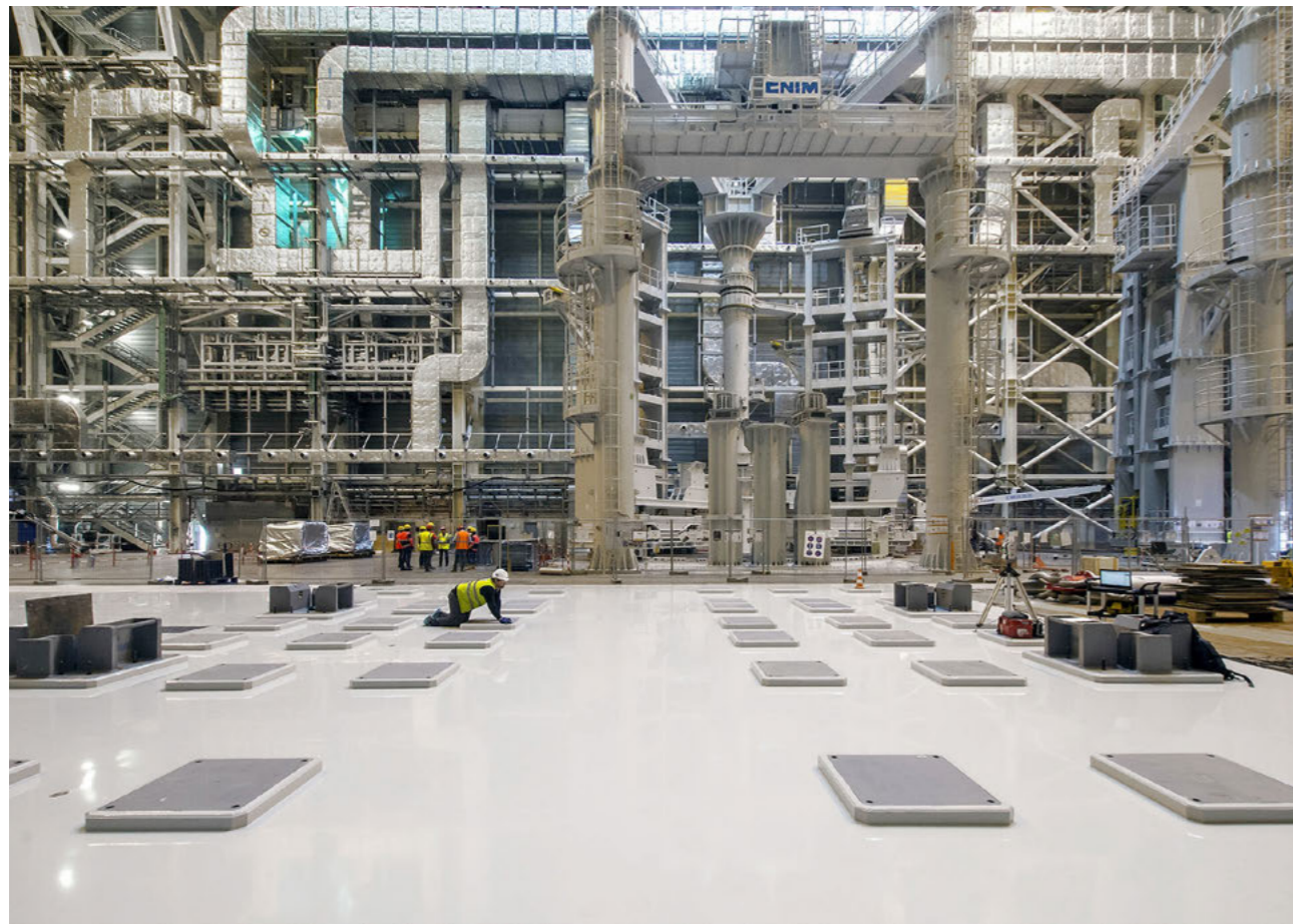
Inside the Assembly Hall, piping and HVAC testing are performed whilst other contractors are coating its 6 500 m 2 floor with epoxy resin, Cadarache, France, October 2019 © ITER Organization
