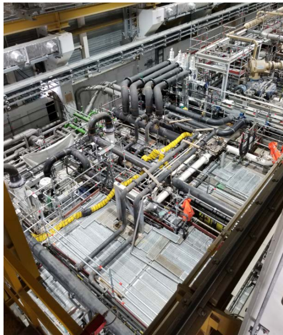
Figure 22: Pre-commissioning of the LN2 Plant and Auxiliary Systems
