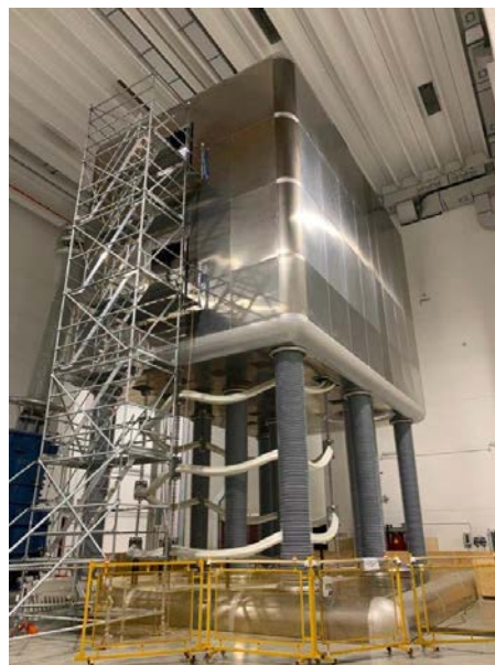
Figure 36: MITICA ISEPS installed inside the HV Deck
