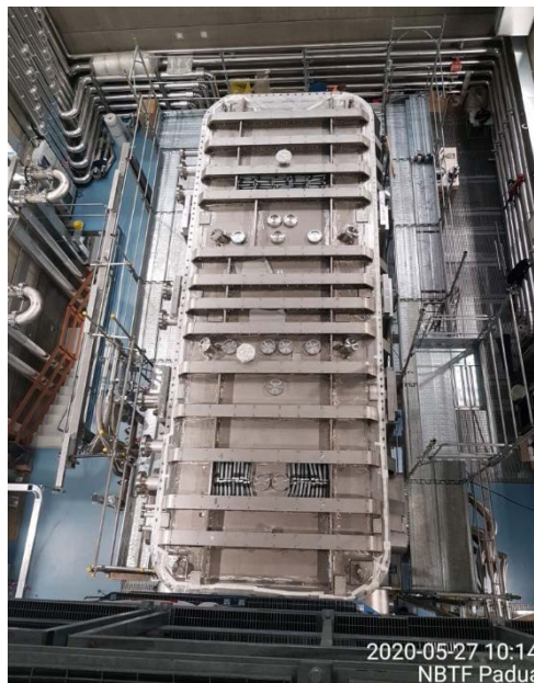
Figure 32: MITICA Vacuum Vessel: installed, site tested and accepted
