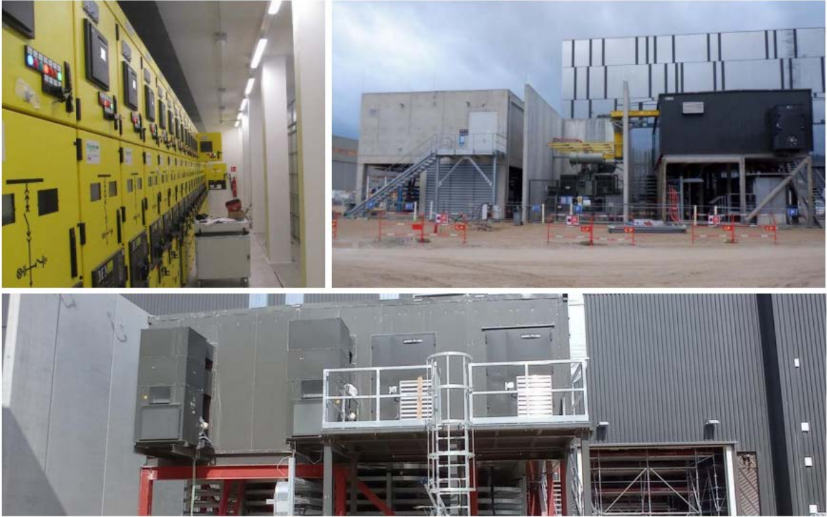
Figure 4: All LC/MV first plasma non-nuclear ready for energization
