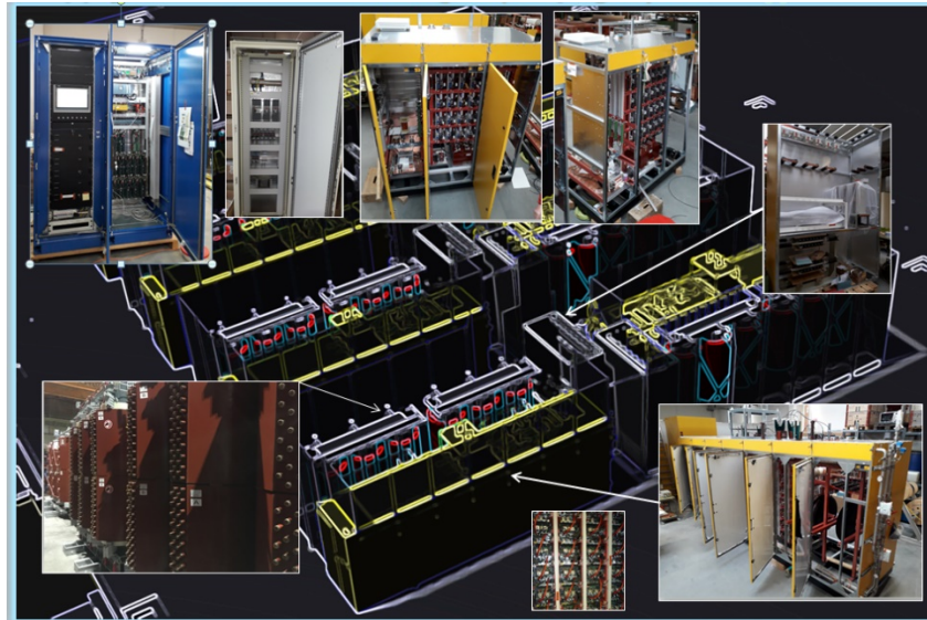
Figure 45: EC Power Supply set#2 delivered to Cadarache
