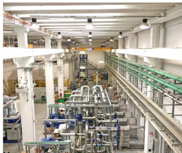
Figure 28: NBTF cooling system: installed, site tested and accepted
