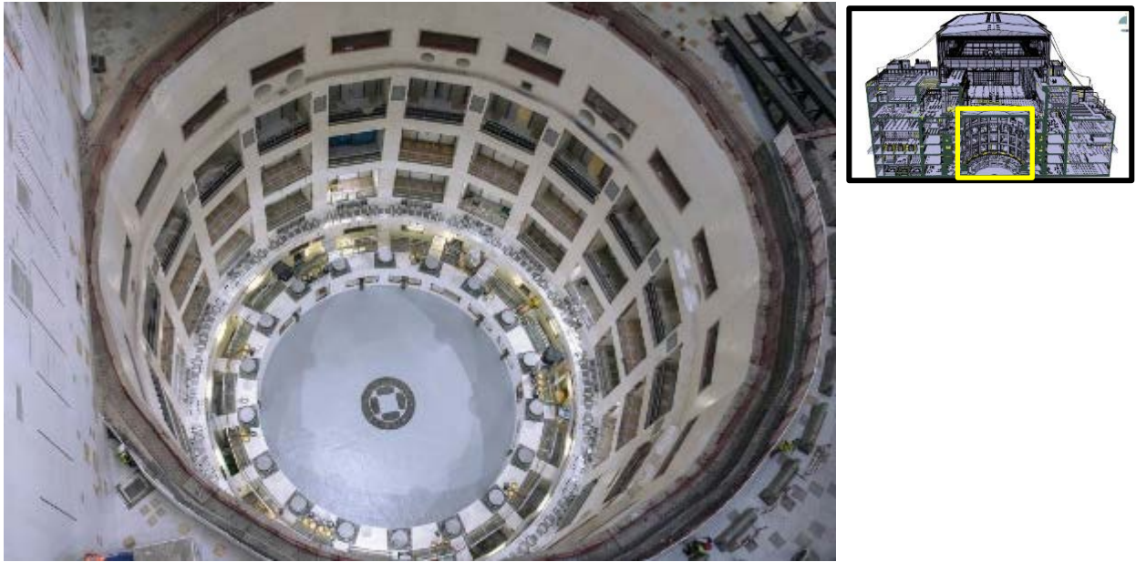
Figure 2: Bioshielded, Concrete Crown and Pit Completed and handed over to IO ready for Cryostat Base lifting
