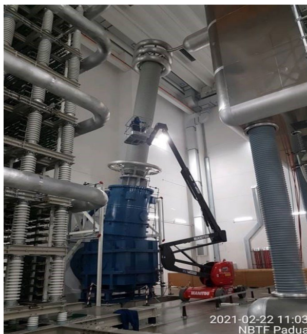
Figure 23: The high voltage bushing connecting the insulating transformer to the high voltage deck of the MITICA power supplies, during the integrated tests
