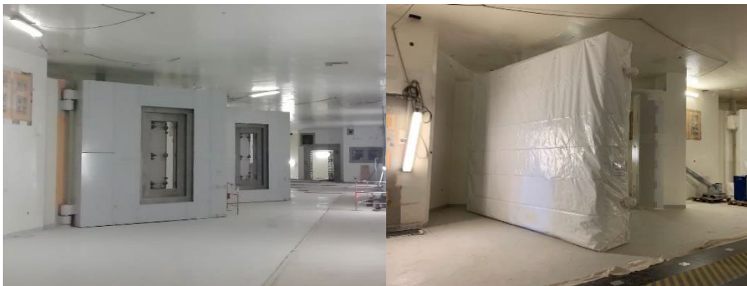
Figure 3: Heavy Nuclear Doors (HND's) before and after installation of cocooning - all transferred to IO in October 2021.
