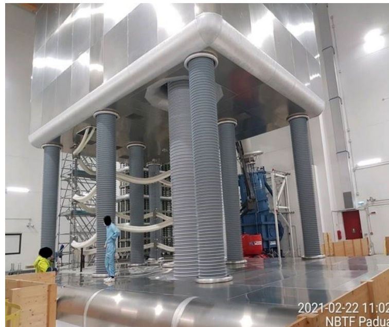
Figure 22: The high voltage deck of the MITICA power supplies during the integrated tests
