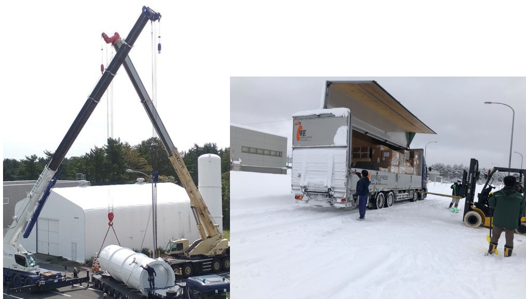
Figure 31: Left, installation of the 2nd buffer tank for the cryomodule cryoplant. Right, delivery of the superconducting solenoids for the cryomodule
