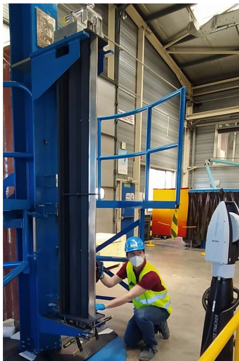
Figure 15: Giacomo Calchi (F4E) completing dimensional checks on the first pumping section for the MITICA cryopump
