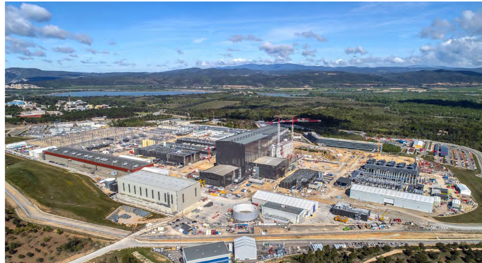
North view of the ITER construction site, Cadarache, France, May 2021. © ITER Organization/EJF Riche
