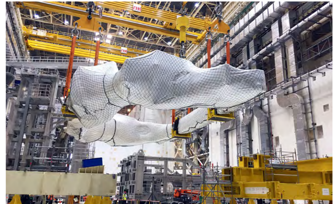
Moving one of Europe's Toroidal Field coils from the transport frame to the storage frame, ITER Assembly Hall, Cadarache, France, July 2021. © ITER Organization
