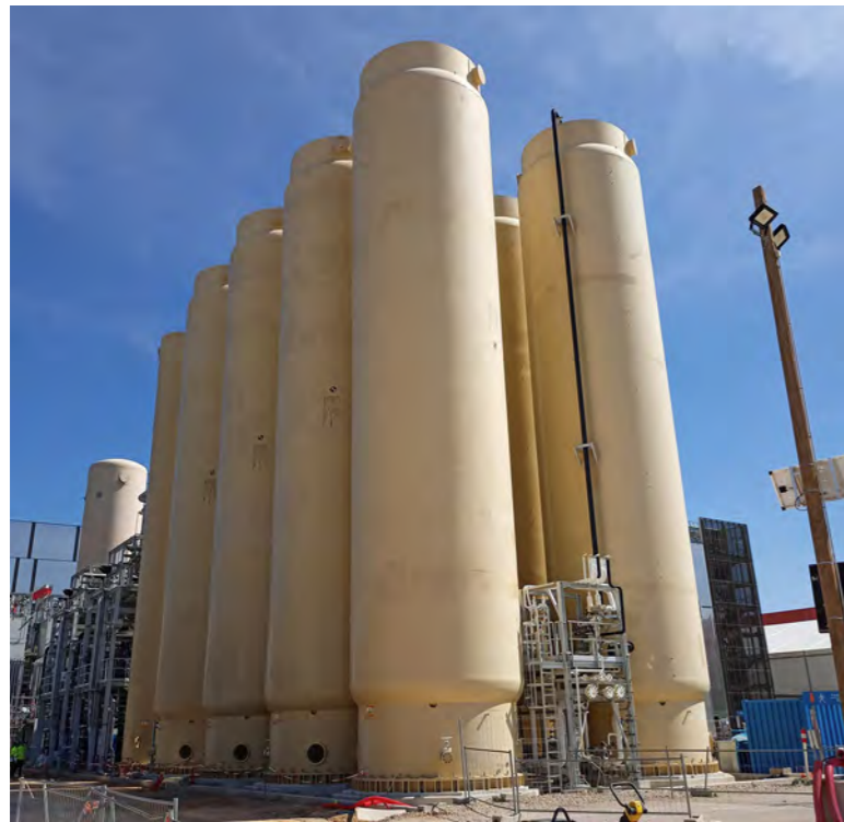
Gaseous helium storages that would be enough to fill 4 million party balloons. Cadarache, September 2021. © F4E
