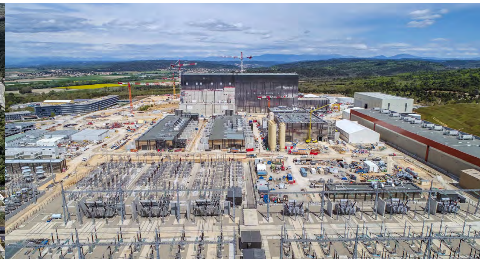
East view of the ITER construction site, Cadarache, France, May 2021. © ITER Organization/EJF Riche
