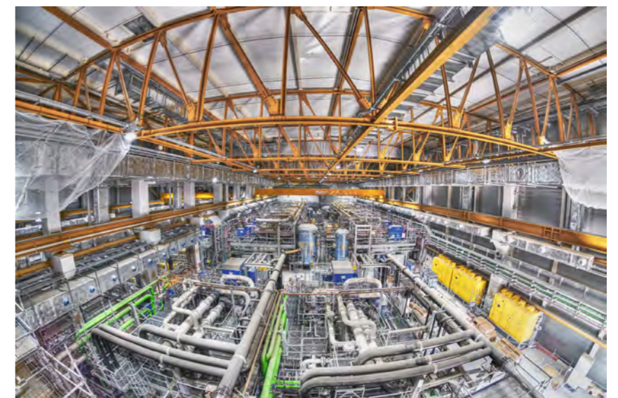
As big as two football pitches, the cryoplant provides cooling fluids for the superconducting magnets, the cryopumps, and thousands of square metres of thermal shielding, Cadarache, March 2021. © Christian Lüning
