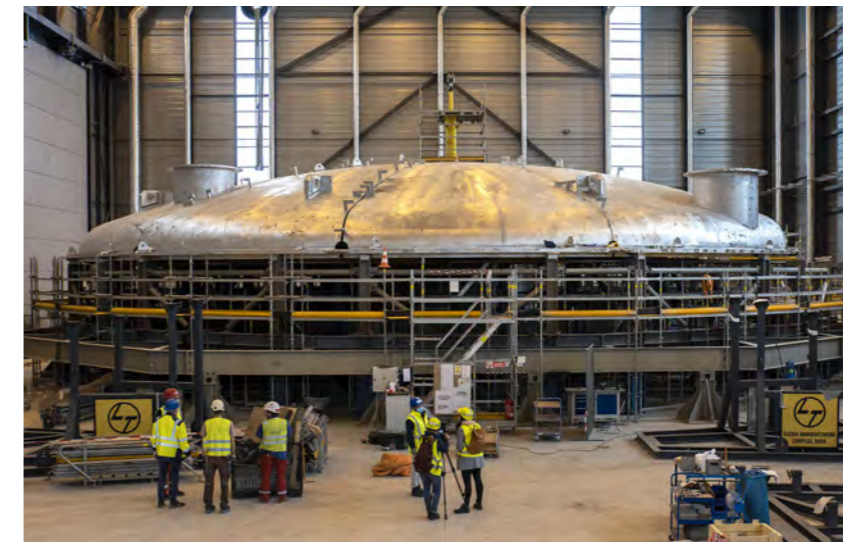
Seven of the 12 segments of the cryostat's top lid have been assembled on the work platform. March 2021 © ITER Organization
