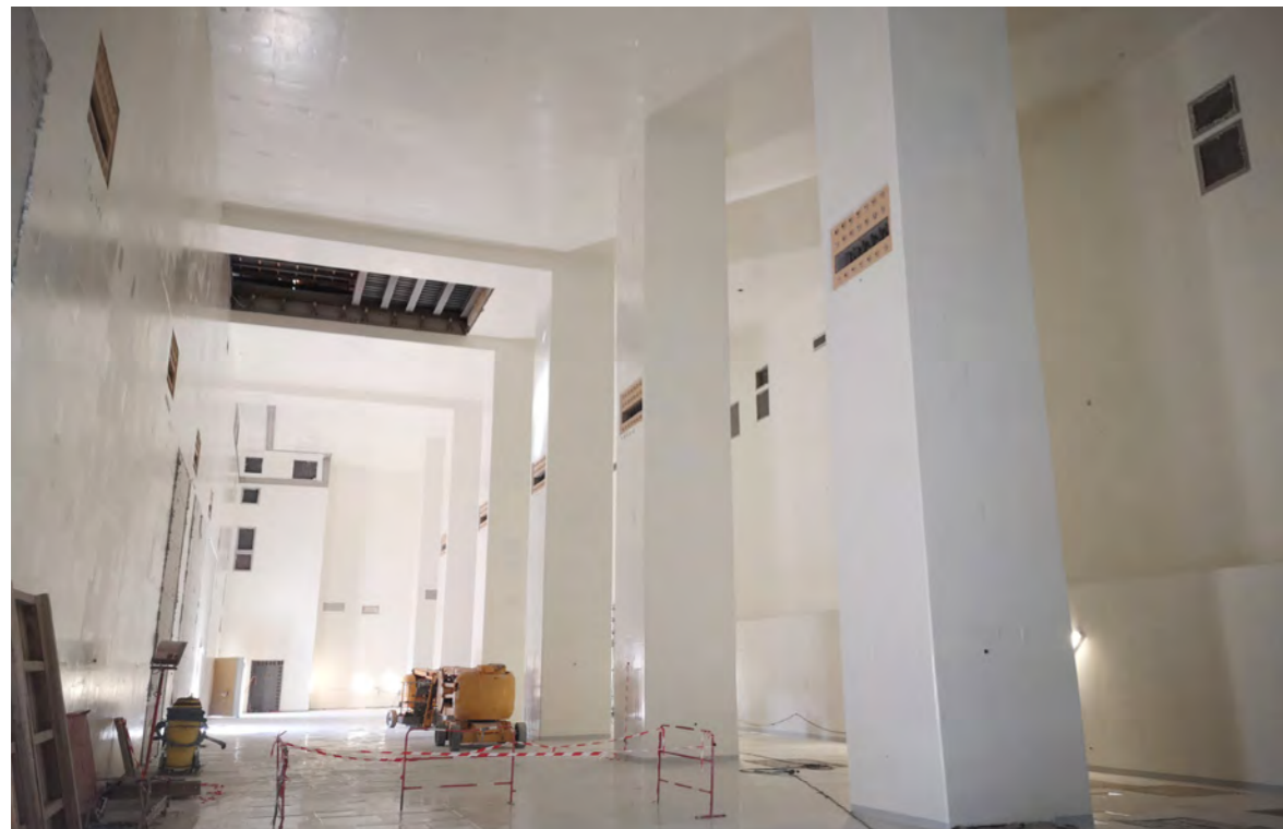
Last layer of paint applied inside the Tokamak building, Cadarache, France, October 2021. © F4E
