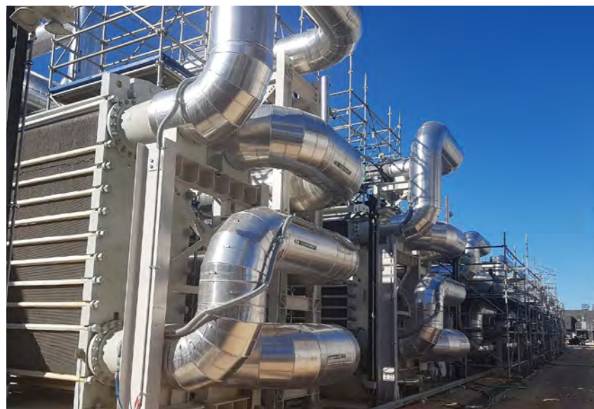
Equipment procured by India has been installed in the 6 000 m 2 Cooling Plant on the northern corner of the ITER site, including heat exchangers as shown in the image. October 2021 © ITER Organization
