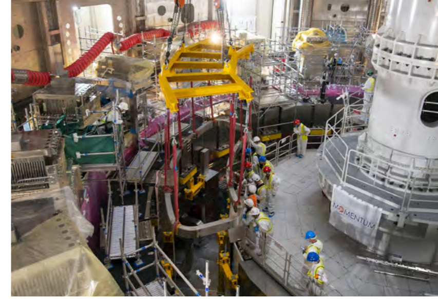
Lowering of correction coil 4 in the Tokamak pit. The space between Poloidal Field coil 5, Poloidal Field coil 6, lower magnet feeders, and staging platforms does not exceed 25 mm. October 2021 © ITER Organization
