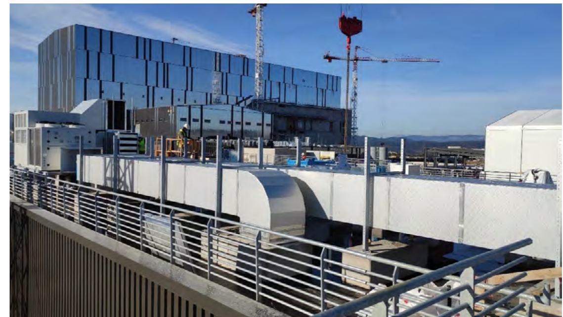
All HVAC equipment installed on the roof of the Tokamak Assembly Preparatory Building, ITER site, Cadarache, France, January 2021. © ITER Organization
