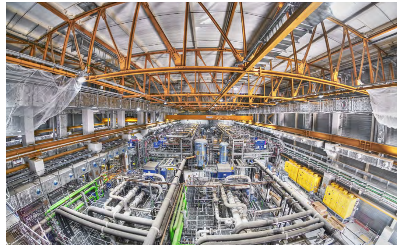
Installation work in the cryoplant nearing completion, ITER construction site, Cadarache, France, June 2021. © Christian Lünig
