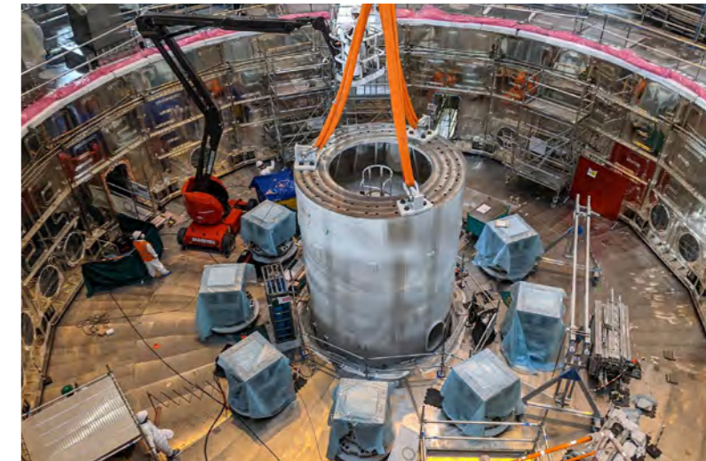
Bottom cylinder of the in-pit assembly tool installed. With a central column and radiating beams braced against the pit walls, the in-pit column tool will support the nine sectors of the vacuum vessel as they are welded together. Cadarache, France, March 2021. © ITER Organization
