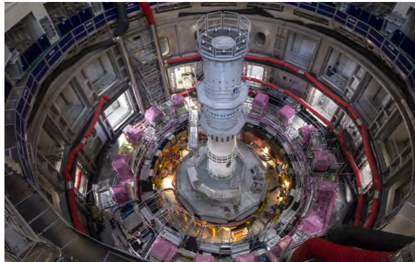
The 30-metre-deep Tokamak pit ready to receive its first 40-degree vacuum vessel section. The central column, equipped with ladders and access ports, will be used to reach different levels of the emerging torus. December 2021 © ITER Organization
