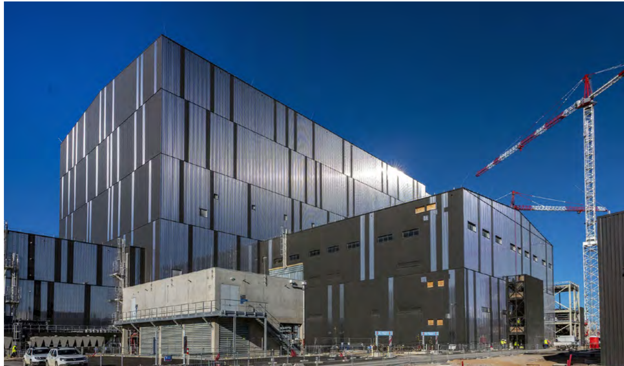
The Radio Frequency Heating Building (on the right) is the radio powerhouse on site, housing all wave-generating equipment for the electron and ion cyclotron heating systems. ITER construction site, Cadarache, France, October 2021. © ITER Organization
