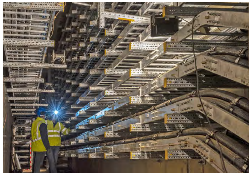
Cables located below the west entrance of the magnet power conversion buildings head in all directions, eventually reaching the four corners of the platform. Procured by China, the cables are delivered in drums and unspooled. February 2021 © ITER Organization
