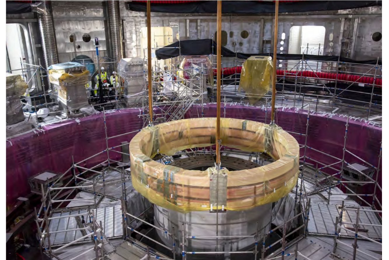
Installation of a set of three spare Pre-Compression Rings in the Tokamak pit, July 2021. Two other sets of three rings will hold tightly the Toroidal Field coils at top and bottom against any expansion forces during operation. © ITER Organization
