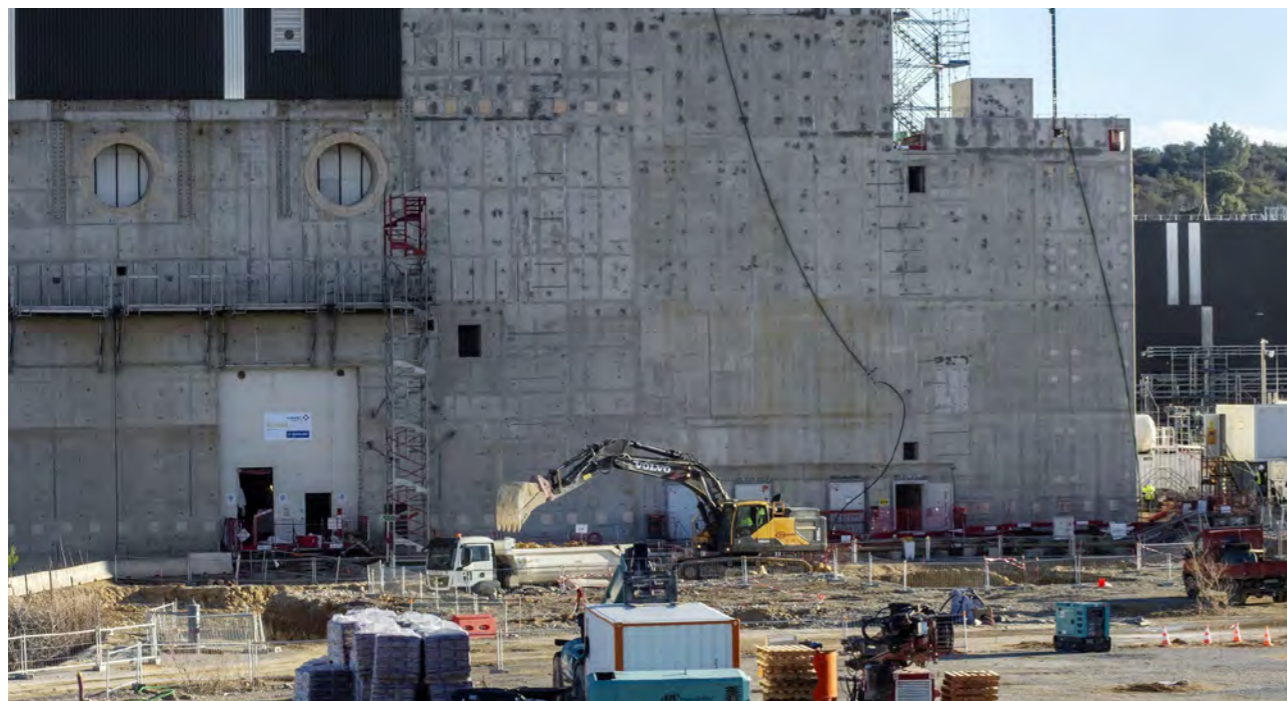
On a level area in front of the Tokamak Complex, excavation works started for a series of buildings that will be dedicated to the power supply of the ITER Neutral Beam heating system, ITER construction site, Cadarache, France, January 2022. © ITER Organization
