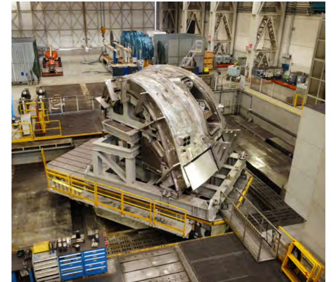
Placing on the jig in the factory of Mangiarotti, poloidal segment 4, manufactured by Mangiarotti, Italy, June 2021. The component is part of sector 5 of the ITER Vacuum Vessel manufactured in Europe. © F4E
