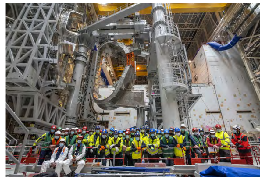
Sector 6 of the ITER Vacuum Vessel, supported by a radial beam above, safely docked in the sector sub-assembly tool, April 2021 © ITER Organization
