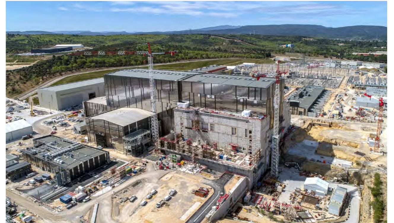
West view of the ITER construction site, Cadarache, France, October 2021. © ITER Organization/EJF Riche
