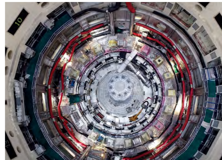
Aerial view of ITER Tokamak pit capturing components, tools, staging platforms and equipment. Cadarache, France, October 2021. © ITER Organization
