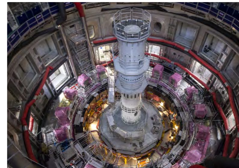
The central column of the in-pit column tool is in place. The nine radial beams will arrive next to support a vacuum vessel sub-assembly. Cadarache, France, December 2021. © ITER Organization
