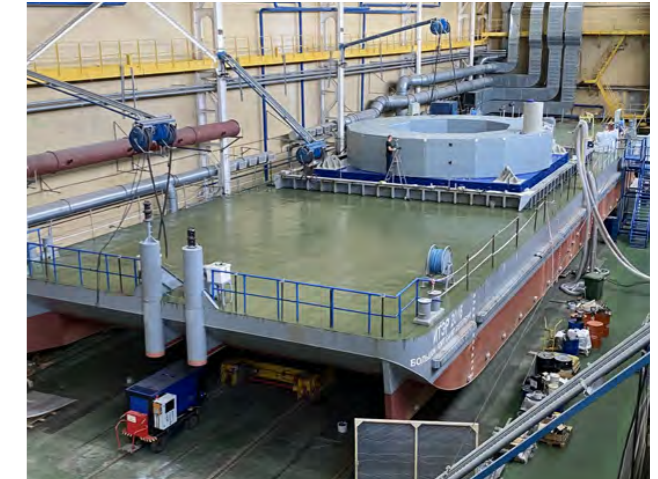
PF1, ITER's smallest Poloidal Field coil, on a barge in order to be transferred to a ship to begin the journey to ITER. July 2022 ©ITER Organization
