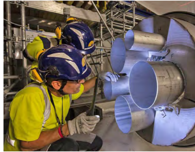
Procured by India, manufactured by INOX-CVA in India and Air Liquide in France, cryolines are high-tech, vacuum-insulated components that host several multi-process pipes transporting different cooling fluids in and out of the ITER Tokamak. October 2022. ©ITER Organization
