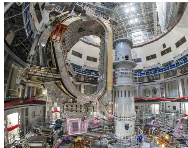
First sub-section of the ITER plasma chamber out of tooling and lowering it into the machine well. May 2022. ©ITER Organization
