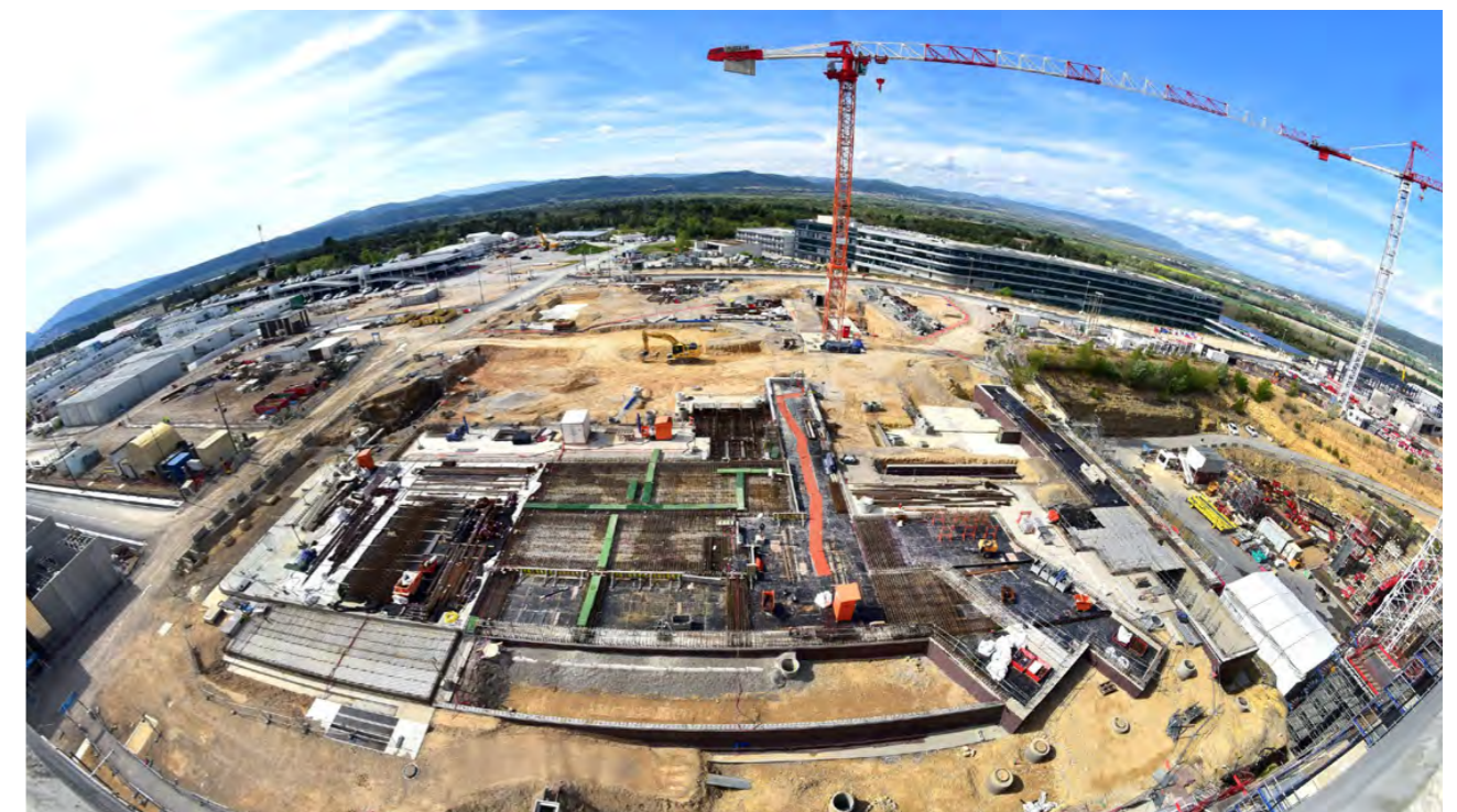
From the roof of the Diagnostics Building, we are looking directly down at the site of the future ITER Neutral Beam Power Supply buildings, currently under construction by F4E contractors. April 2022. © ITER Organization
