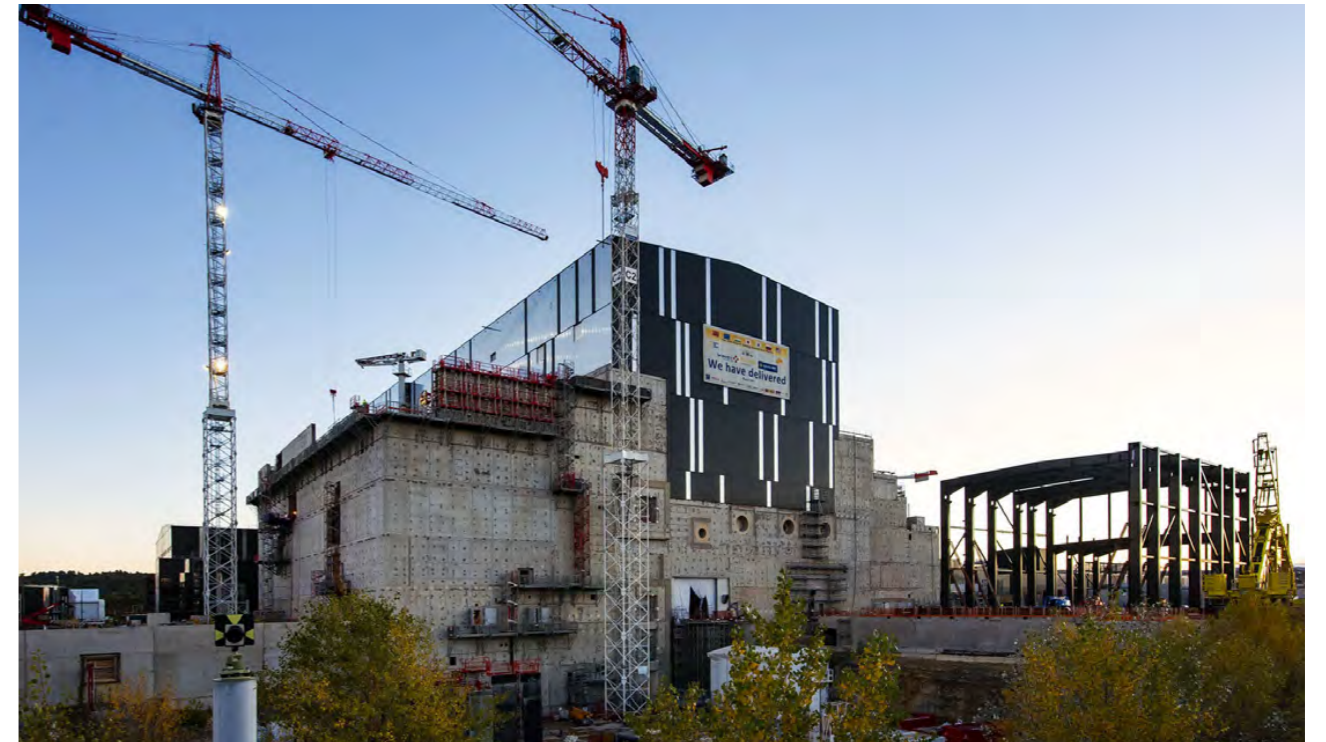
Last level of concrete poured at Level 5, bringing the structure to full length. December 2022 © ITER Organization
