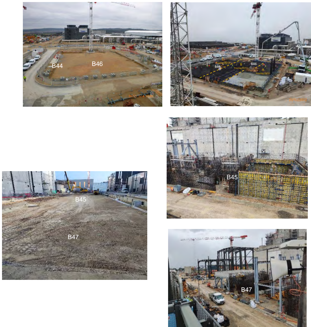
Figure 3: TB13 (Ansaldo - Monsud) B44, B45, B46 and B47 Power Supply and Distribution Buildings work status in Jan 2022 (left) versus November 2022 (right) Photos: © ITER Organization
