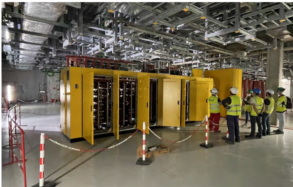
Figure 35: Inspection of the two first Main High Voltage Power Supplies (MHVPS) installed in the ITER Radio Frequency (RF) Building, Cadarache, France, April 2022
