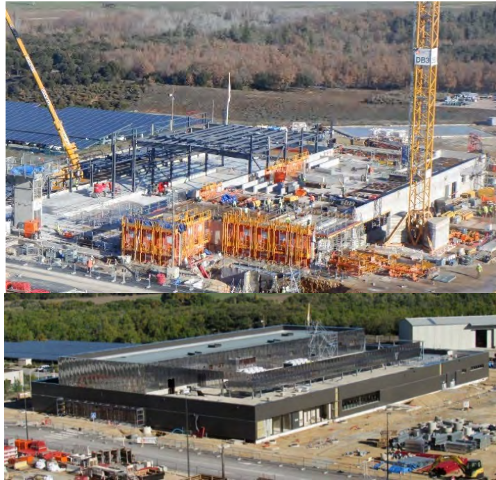
Figure 4: TB12 (Demathieu Bard) B71 Control Building North work status in December 2021 versus November 2022
