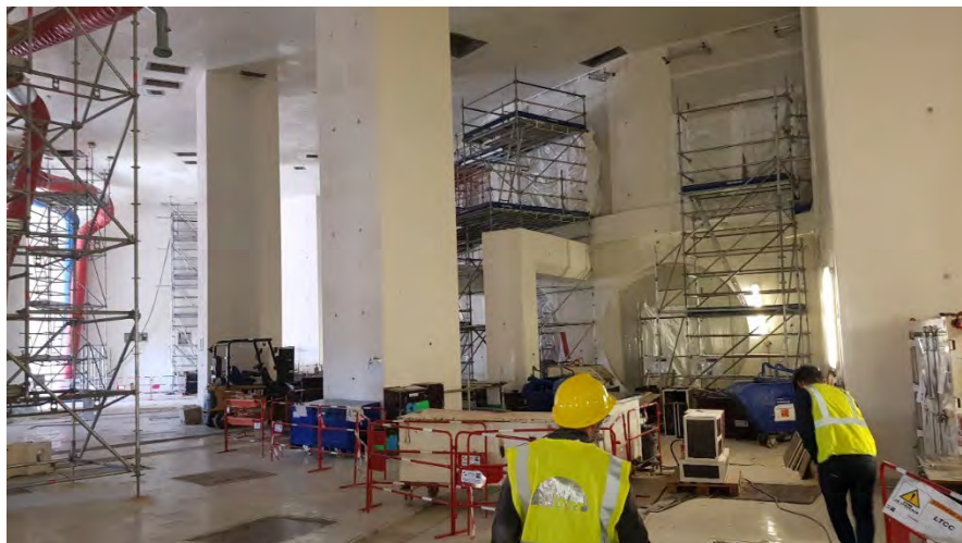
Figure 53: Supervision Activities on the ITER Neutral Beam cell for preparing dimensional inspection activities for reconstructing the as-built of the Cell and prepare the metrology network installation
